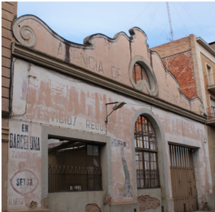
Fig. 5 Industrial site, Clerch i Nicolau Street, architect unknown, Figueres. Source: Esteban Castañer Muñoz
