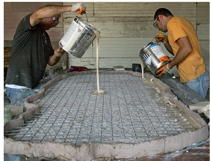
Figure 5 Casting of new fragment backing using RenCast CW 2215 foaming epoxy system. Photo: Elena Kantareva-Decheva, 2011
