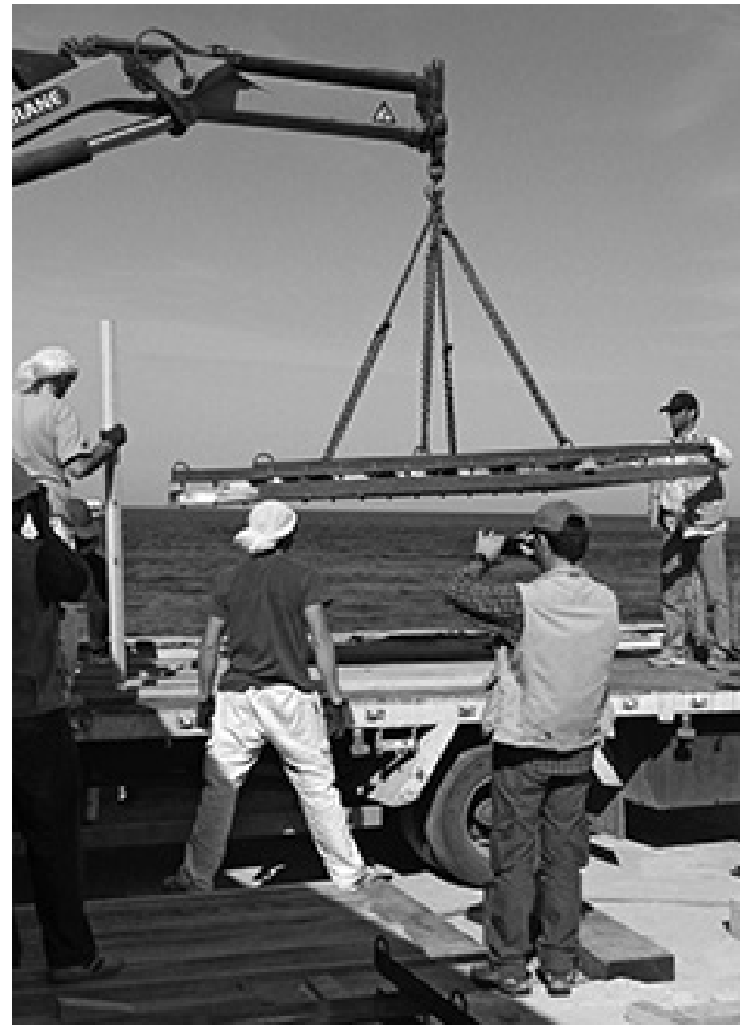
Figure 5 Lifting phase of one of the mosaic panels, showing the crane lifting the made-to-measure metal box. Photo: ISCR Archive
