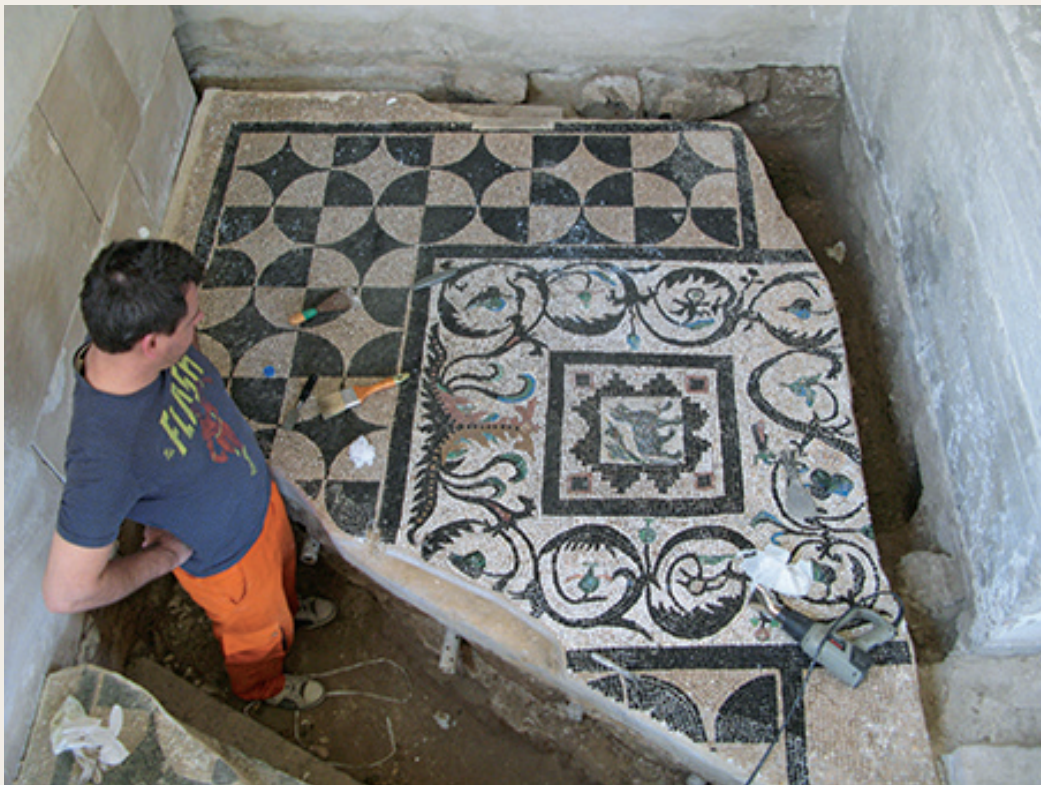
Figure 2 New drainage system with pierced tubes inserted into the bedding layer. Photo: E. Parandowska
