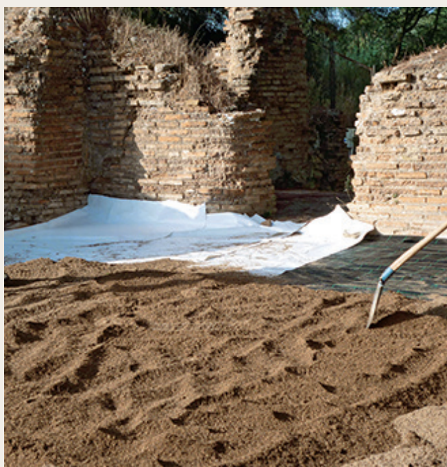
Figure 4 Application of the new reburial materials on the central mosaic of the Kladeos Bath complex. © Hellenic Ministry of Culture and Sports
