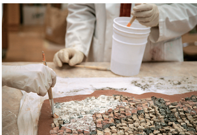
Figure 4 Application of the bedding mortar to the Emona mosaic. Photo: Documentation RC ZVKDS
