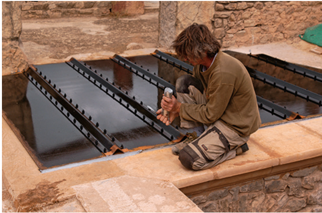
Figure 6 New cover over the missing vaults in the House of the Hunt (Maison de la Chasse) at the site of Bulla Regia, Tunisia. Photo: Gionata Rizzi
