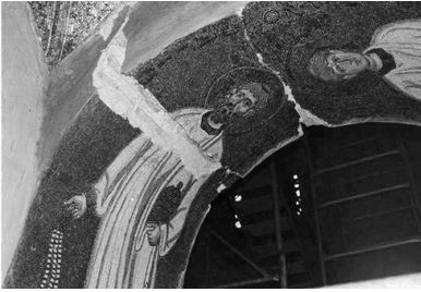
Figure 1 Large loss of tessellatum area after the earthquake. Photo: © Hellenic Ministry of Culture and Sports
