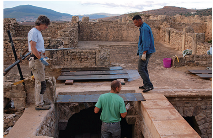
Figure 7 Installing the new cover over the missing vaults in the House of the Hunt (Maison de la Chasse) at the site of Bulla Regia, Tunisia. Photo: Gionata Rizzi
