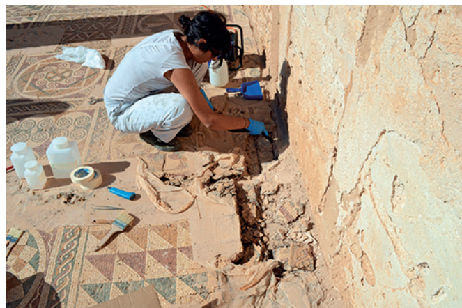
Figure 3 Removal of materials used during earlier work; iron rods in the concrete that have caused severe deformation and cracks are visible.
