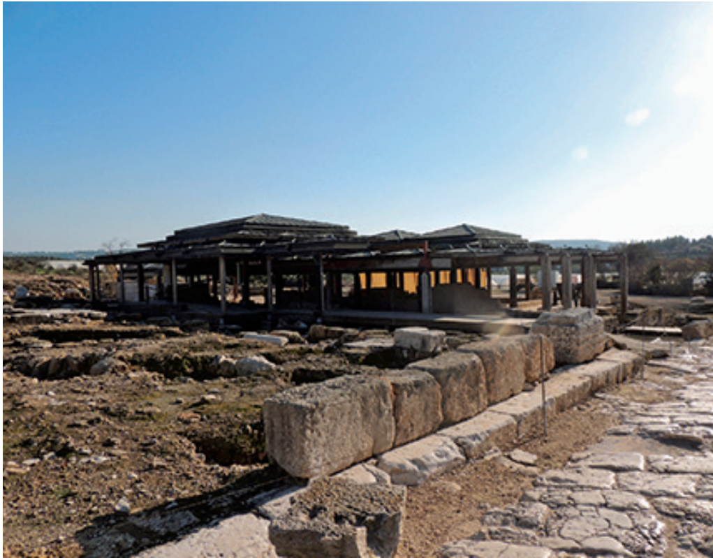
Figure 5 View of the open shelter over the Nile Festival building next to the cardo. The modular roof is composed of a complex system of pyramids made of fiberboard covered with copper sheets.
