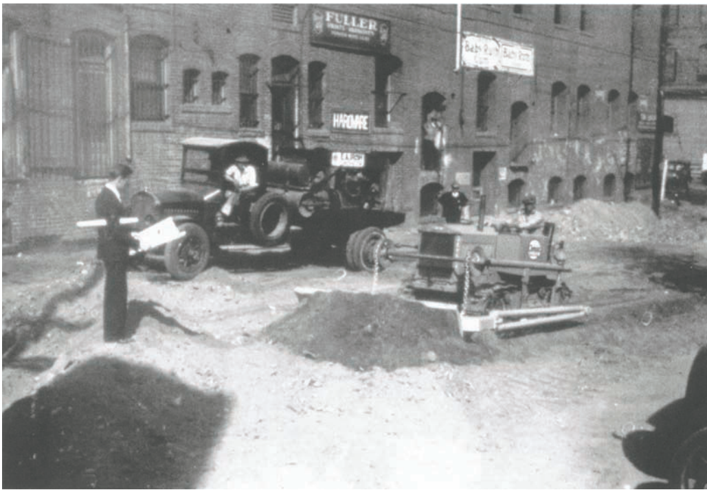
Engineer from the Los Angeles Department of Water and Power checks plans for the grading of Olvera Street during its renovation in late 1929 and early 1930.
