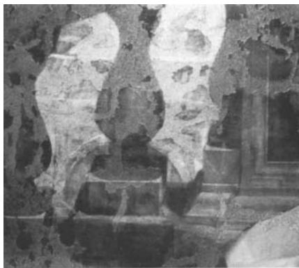
FIG. 9 Detail of balustrade after restoration. Note difference in level between the original layer and the reconstructed areas.
