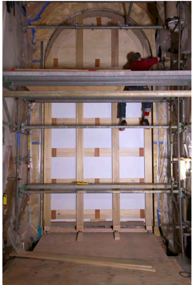
Figure 12.3 The mural faced with support panels and stiffening wood members. Image: Gianfranco Pocobene Studio
