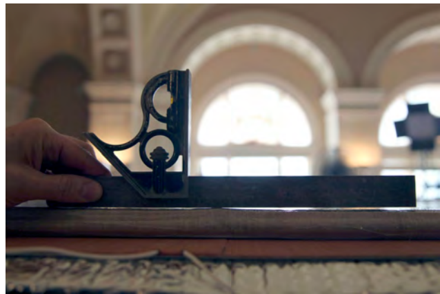
Figure 12.5 A straight edge placed on the failed structural seam of the aluminum honeycomb panel, revealing the protrusion of the aluminum panel skin. Image: Gianfranco Pocobene Studio
