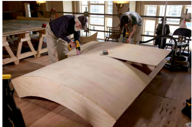
Figure 12.6 Conservators constructing a curved form to be used to roll the partially adhered section of the mural off of the aluminum honeycomb panel. Image: Gianfranco Pocobene Studio
