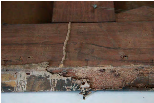
Figure 61.3 Damage due to termite attack to back side of stretcher bar. Image: Victoria Memorial Hall, Kolkata, India
