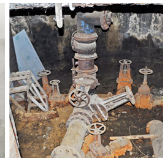
[pic.17] Water pipes in the basement. From the archive of RDNK surveys.
