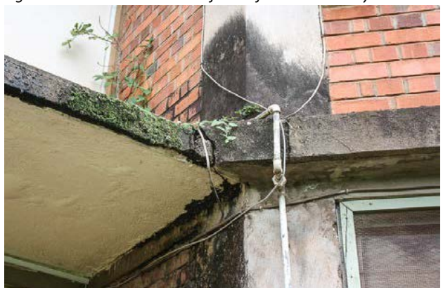
Figure 70 – Inadequate drainage has led to concrete saturation
