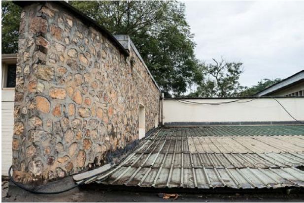
Figure 89 –the failure of flashings between building components
