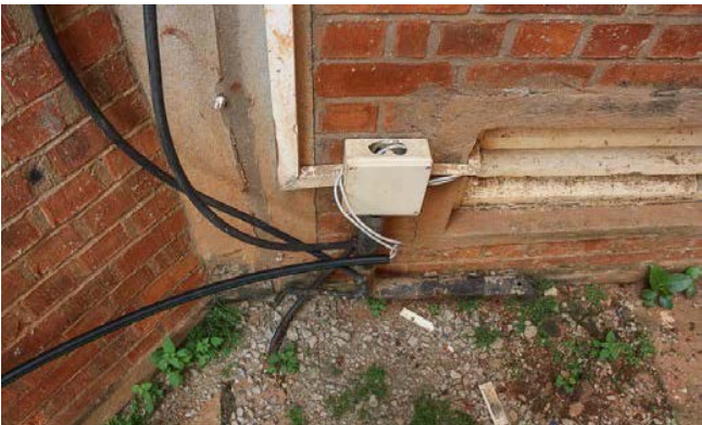
Figure 124 – Exposed electrical at the building exterior
