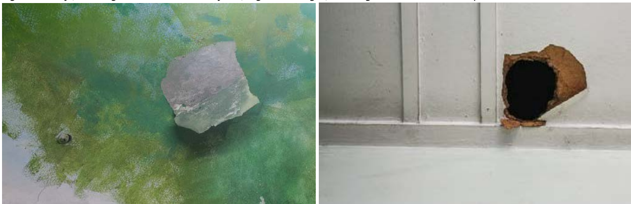
Figure 103 left, peeling paint at the mural in the Natural History Gallery Figure 104 left, holes in ceiling boards in the office
