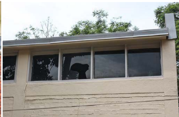
Figure 98 additional broken glass in the north wing
