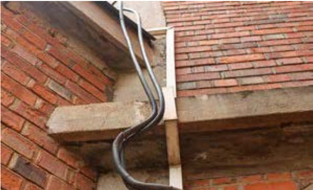
Figure 126 – Unsupported electrical cables
