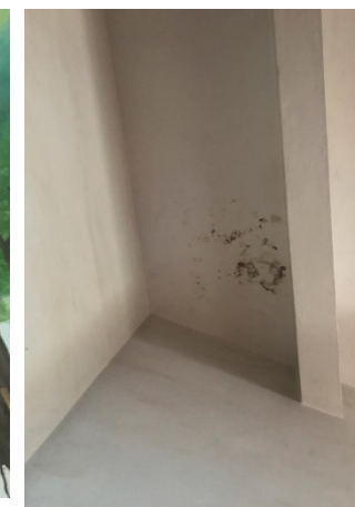
Figure 149 – Stained ceiling in the ethnography section due to leaking roof
