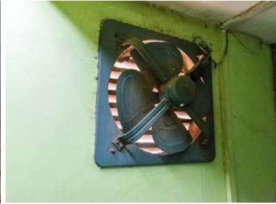
Figure 123 – ventilation fans inoperable
