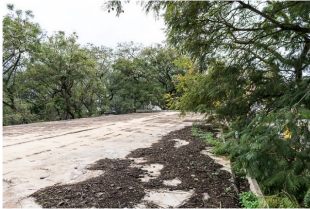
Figure 90 –trees and lack of maintenance contribute to roof failure
