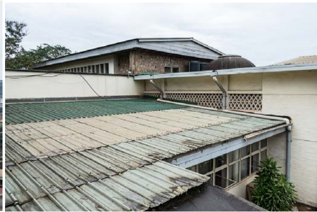
Figure 88 –The ad hoc repairs over the oldest part of the building at the entry
