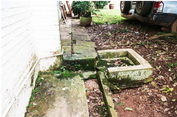
Figure 66 – missing drainage covers and growth of mold
