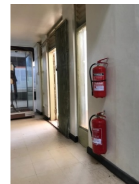
Figure 151 – Fire extinguishers reduce the potential impact of a fire.
