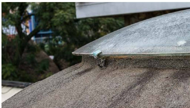
Figure 76 –various metal clips have corroded and failed
