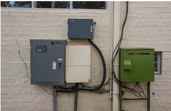
Figure 125 – It is unknown if the electrical panels are adequately sized
