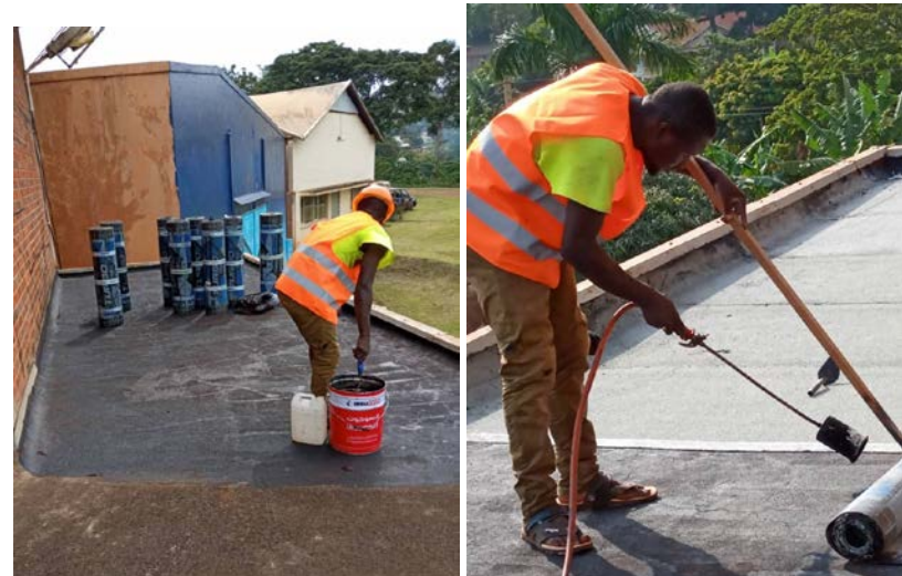
Figure 139 – Left and right roof repairs at the library wing and over the diorama (Denis, 2021)
