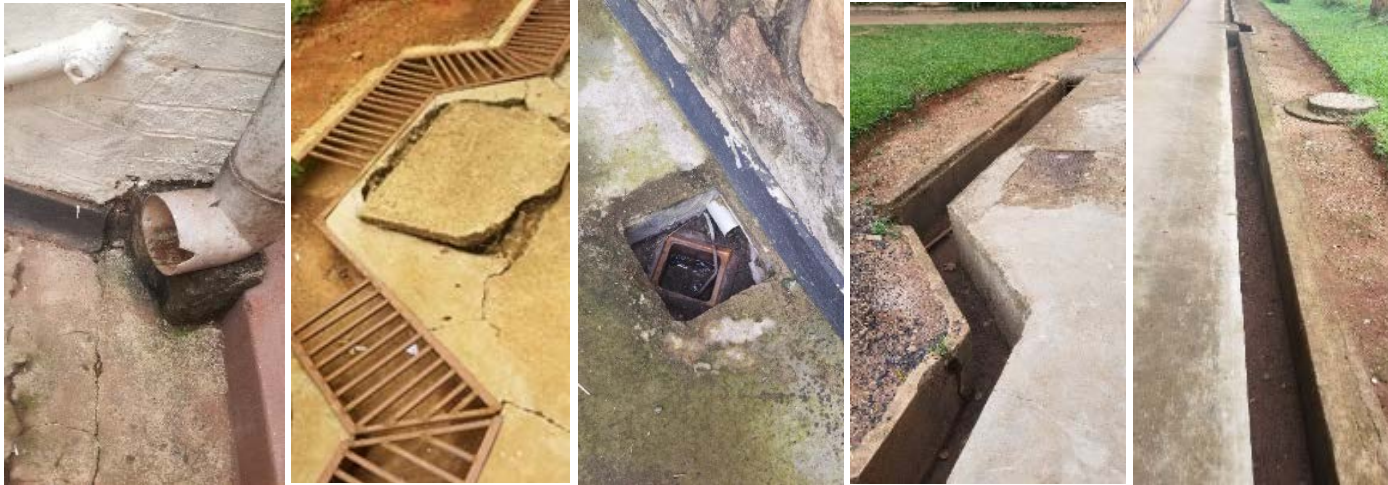
Figure 134 – Leaking drainage pipes, Figure 135 – Incomplete pipe network, Figure 136 defective covers Figure 137, Open drainage channels
