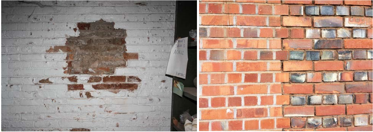
Figure 73 –excessive dampness and inappropriate paint in the masonry of the basement Figure 74 –a variety of bricks during the extensions were made.
