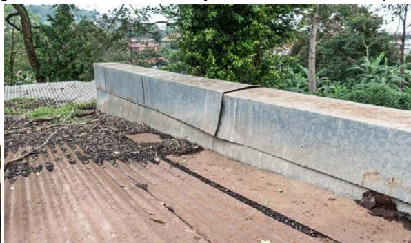
Figure 79 - metal roofs and flashings are also failing
