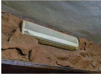
Figure 122 –inoperable phase-change HVAC
