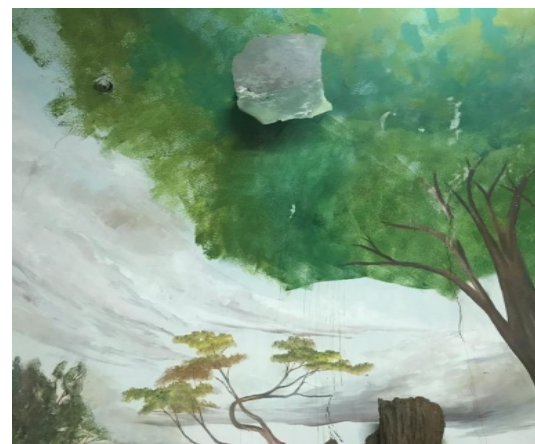
Figure 148 – Cover Cracked and stained ceilings in the diorama section at the Museum. Evident also is the delamination of paint layers.
