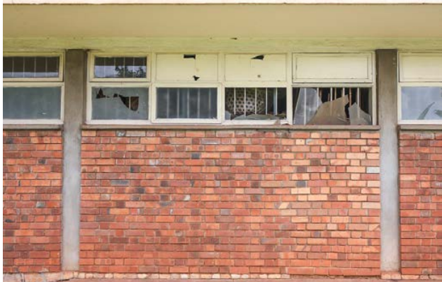
Figure 97 – Broken glass in the store area
