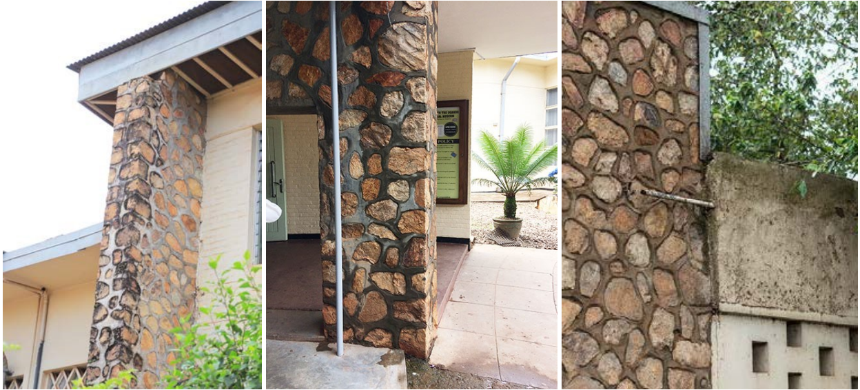
Figure 75 –a variety of issues with the masonry, including water damage, microbiological growth, inappropriate treatment, and poor flashing details
