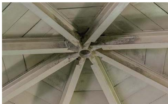
Figure 77 –the metal structure of the South Pavilion is acceptable
