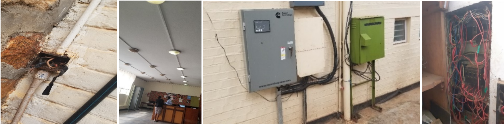
Figure 130 – Exposed socket outlets, Figure 131 – Faulty lighting fittings, Figure 132 – Unsheltered switch gear Figure 133, Exposed connections in the consumer units
