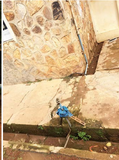
Figure 120 –leaking exterior plumbing
