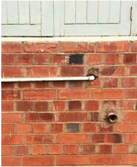
Figure 118 –ad hoc plumbing repairs
