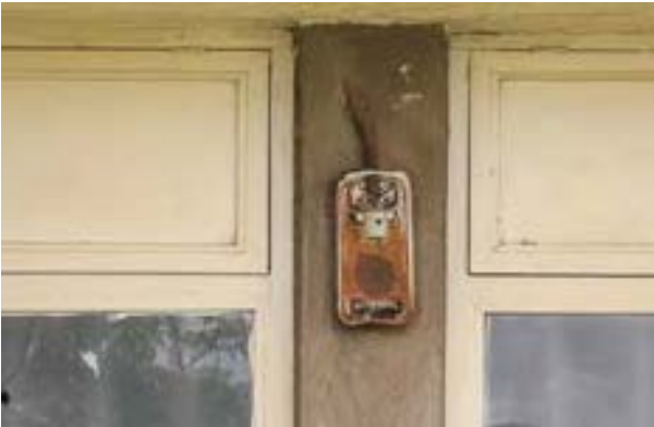
Figure 127 – A number of critical light fixtures have been abandoned
