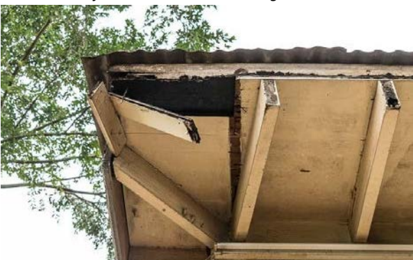
Figure 83 –wooded soffit has failed near the Office Extension
