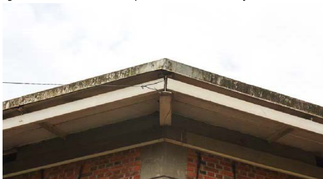
Figure 78 –flashings, clips, and other elements are failing
