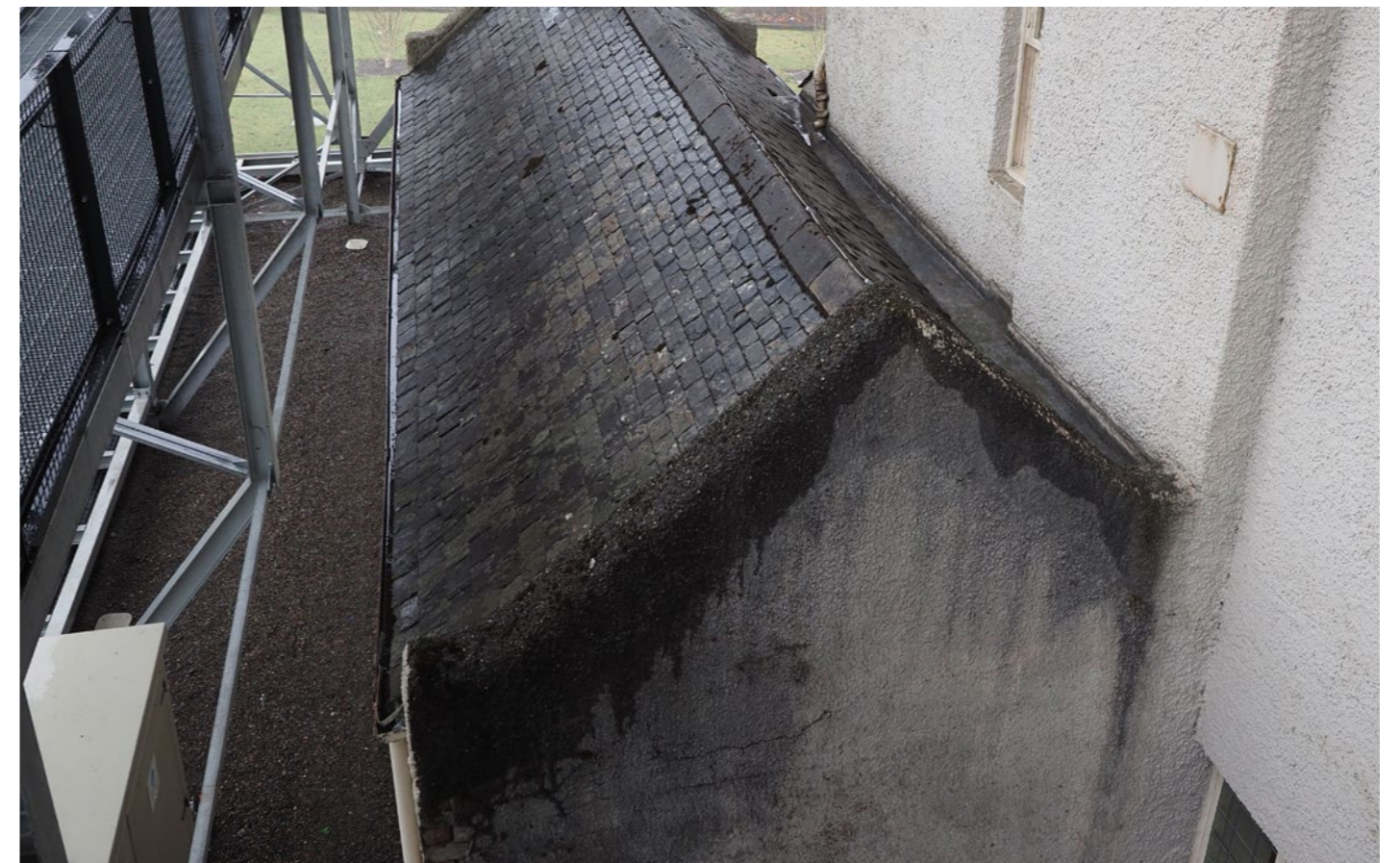
The Box is not fully weather tight and exposed elements of the house continue to be soaked depending on prevailing weather direction
