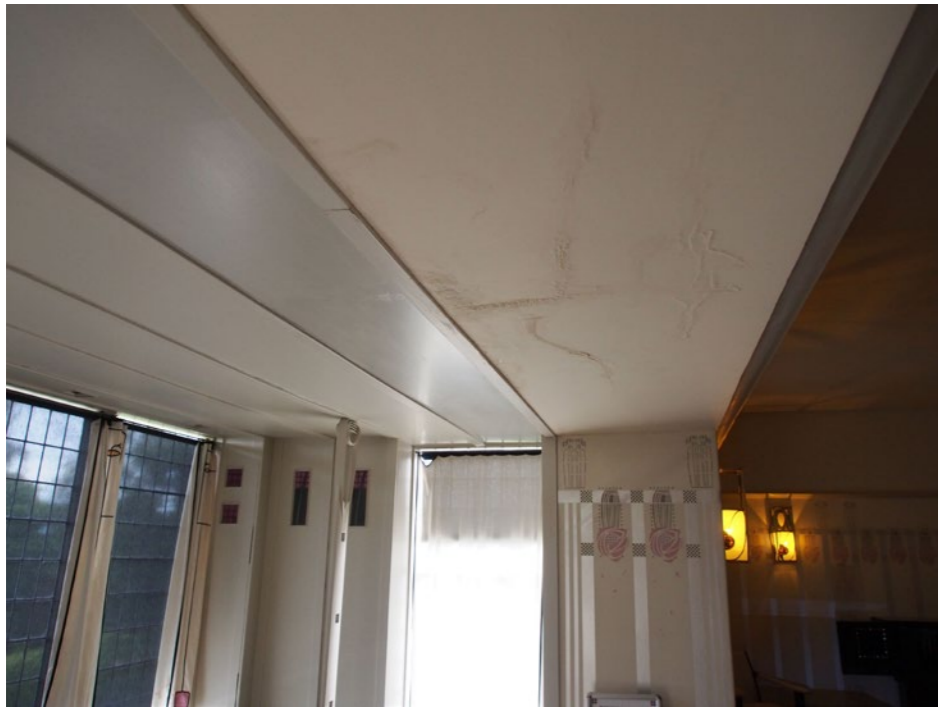
Water ingress and staining above Bay Window of Drawing Room
