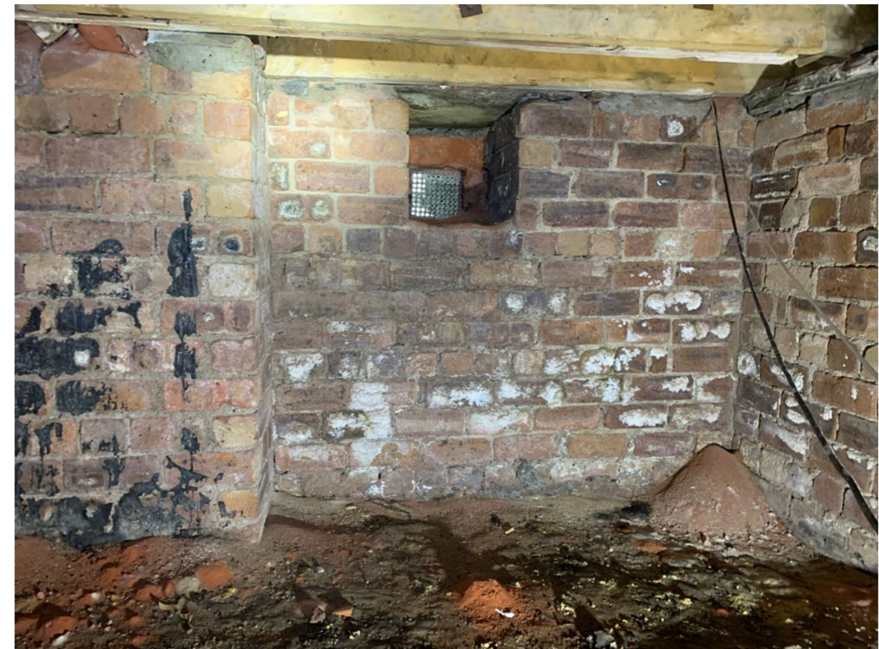
Solum showing piles of decomposed stone and brick from the external walls. Crumbling brick and stone behind internal wall finishes is likely to be forming wet bridges
