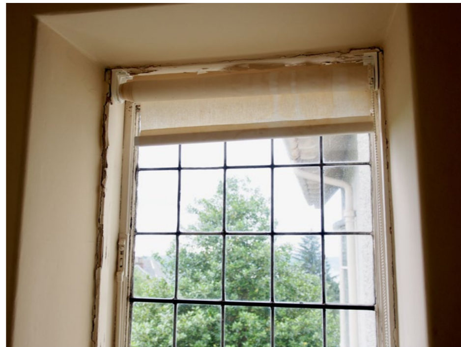
Water ingress and damage around windows
