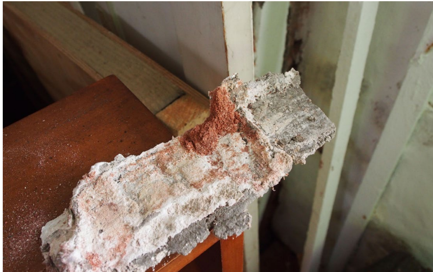
110 Remains of saturated and decomposed brick in East Gable of Attic, 2021
