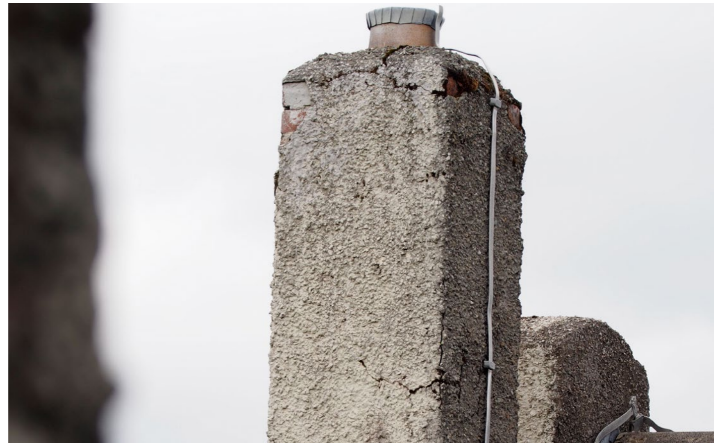
Chimney roughcast spalling
