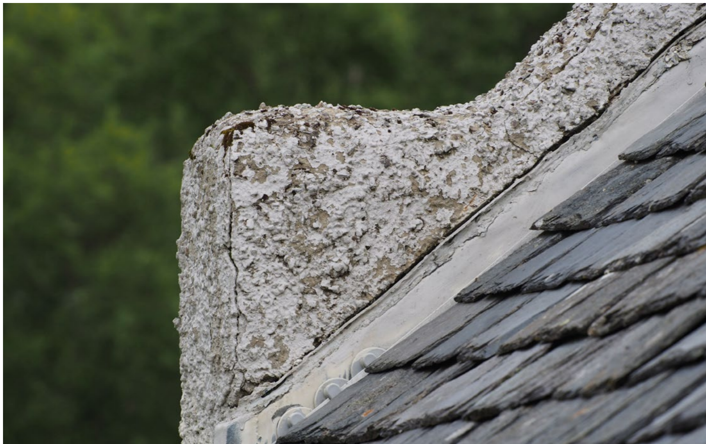
Cracked wallhead weathering and flashings
