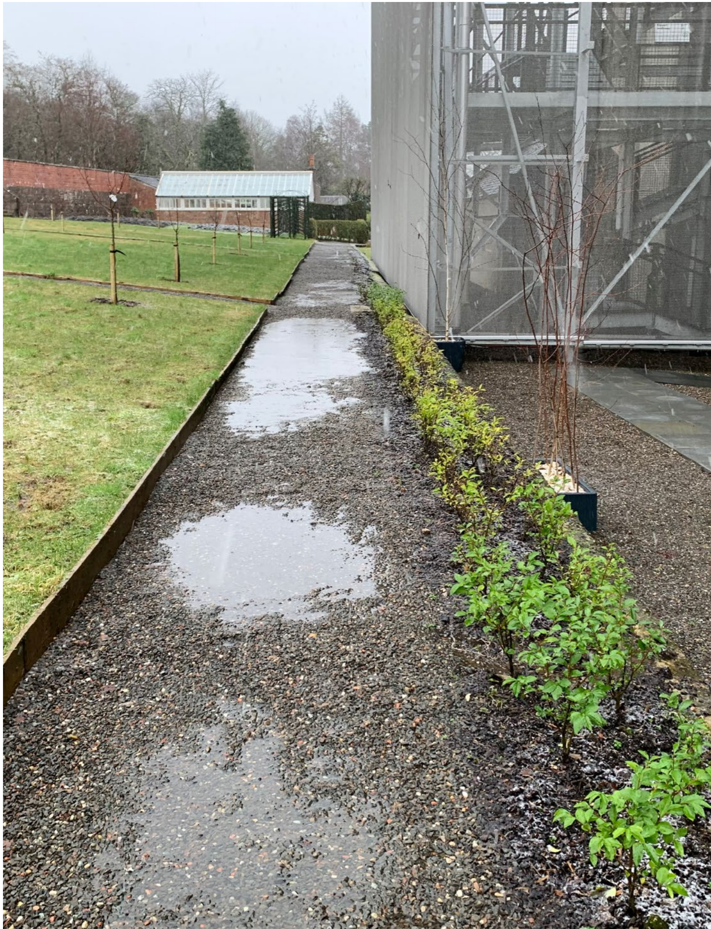
46 Ground water pooling along North Elevation, 2021
