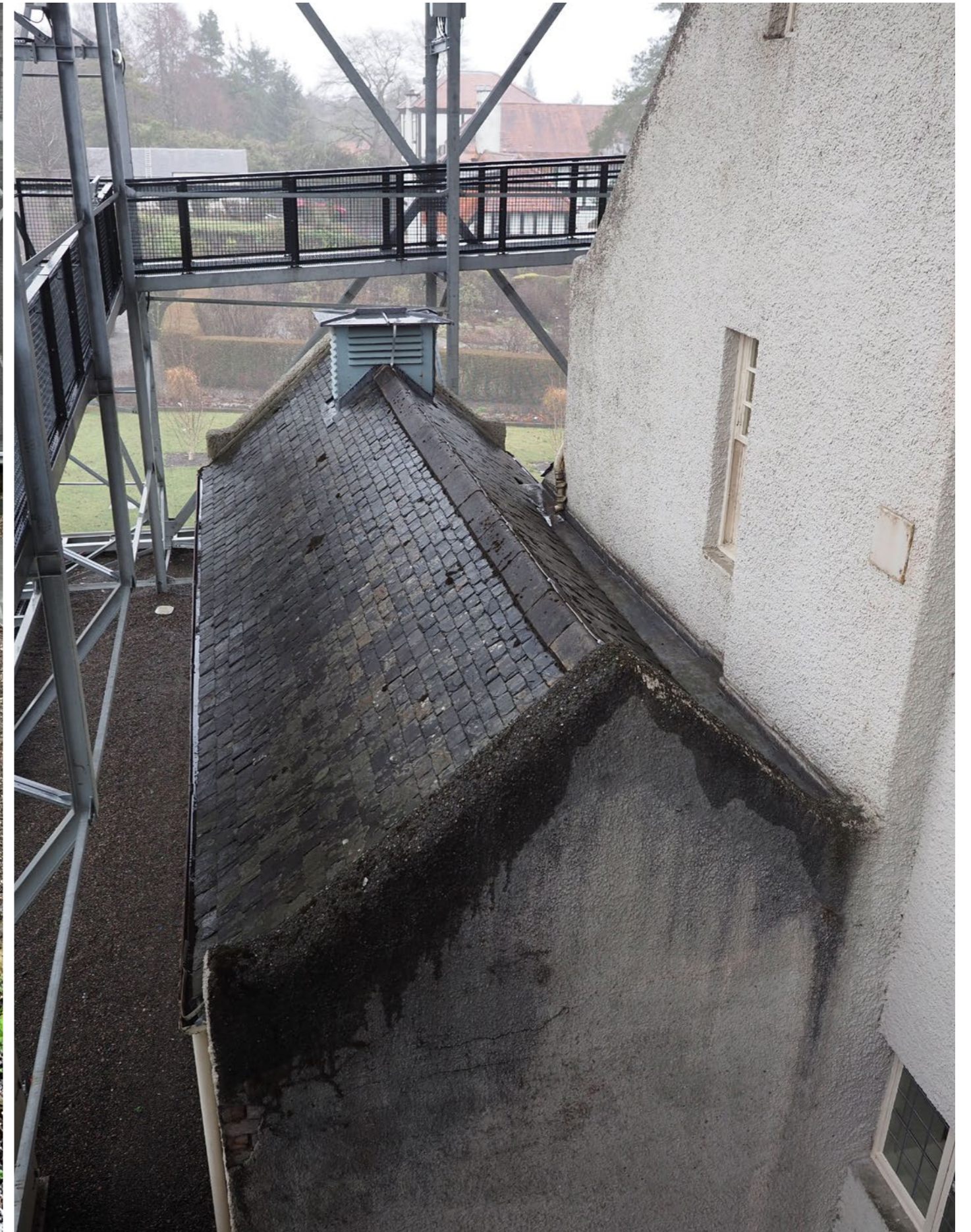
Elements of the building continue to be saturated in bad weather, depending on wind intensity and direction, 2021
