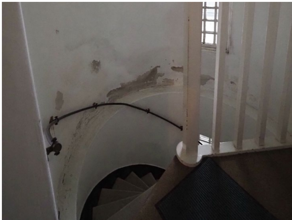
Water ingress and staining in stair tower
