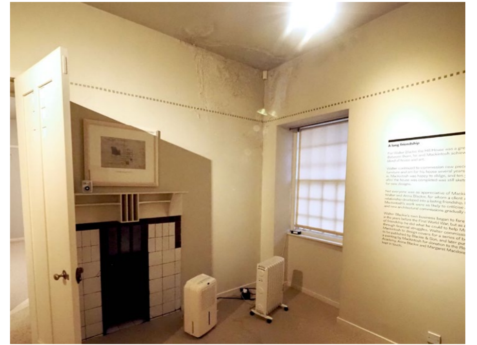
Water ingress and damage, including rot, in Guest Bedroom Dressing Room
