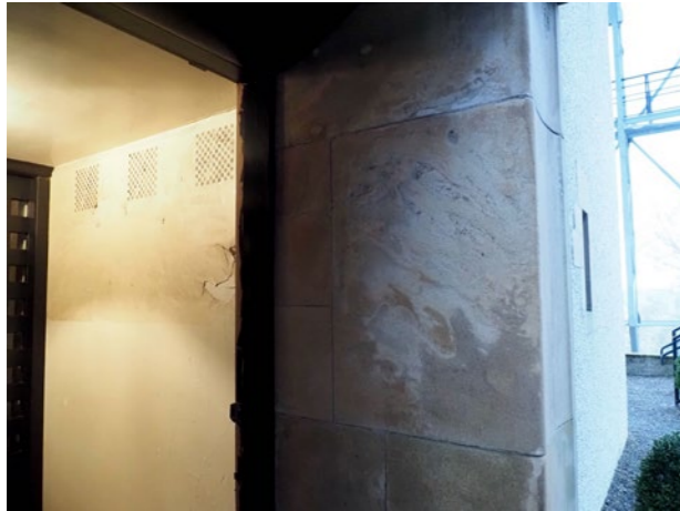
Stonework around entrance showing signs of delamination and efflorescence as a result of being saturated
