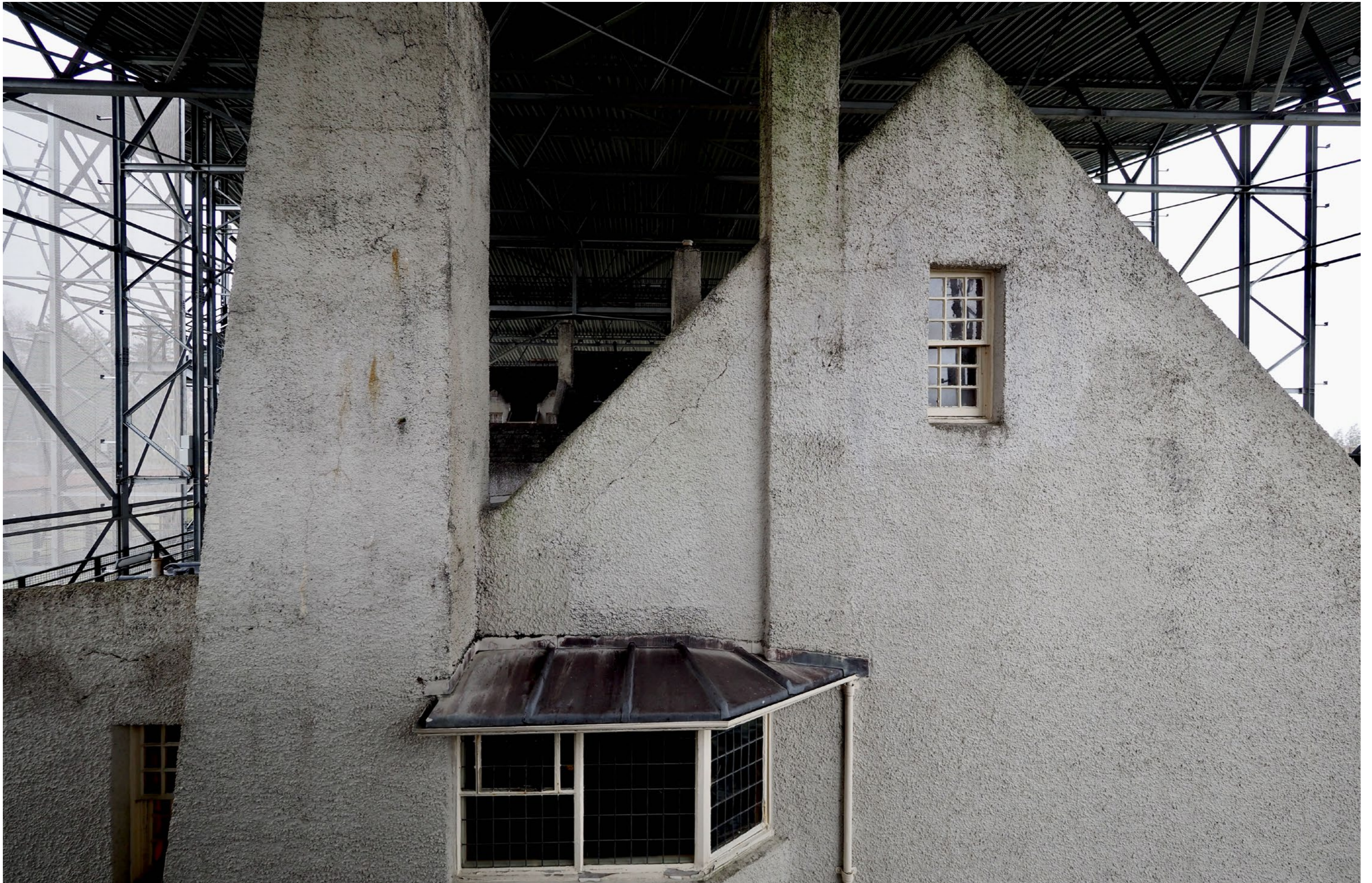
Dryness within Box and build up of dirt are highlighting cracked roughcast and other defects
