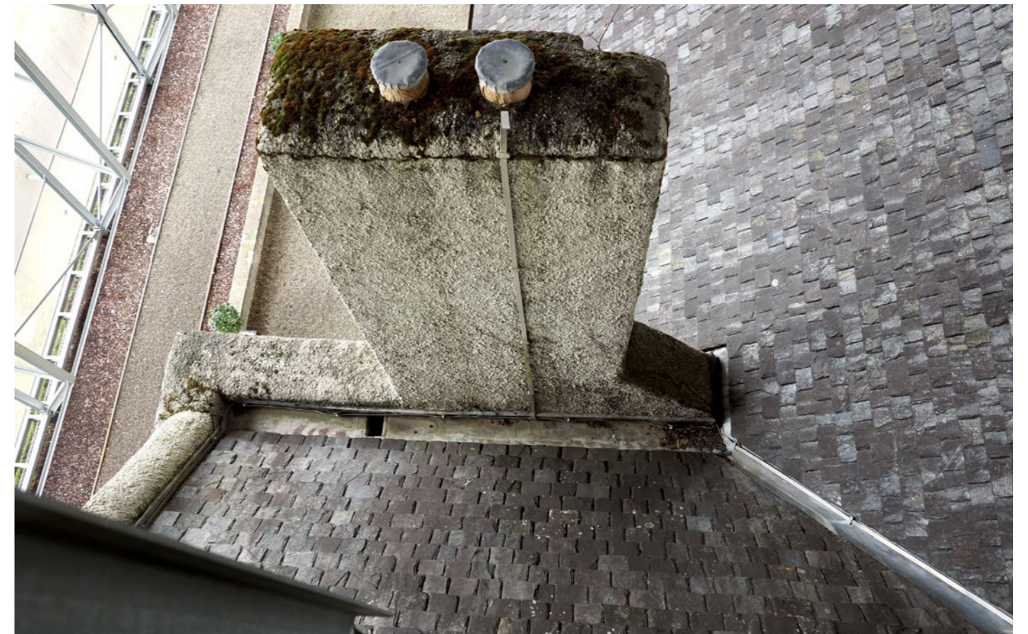
The Box should allow chimney caps should be removed to improve ventilation and drying out of fabric
