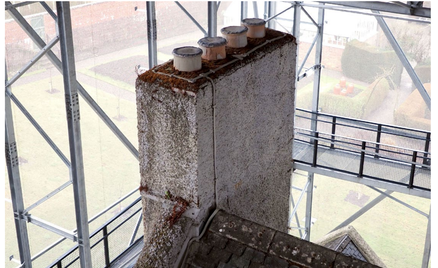
Moss growth and capped flues
