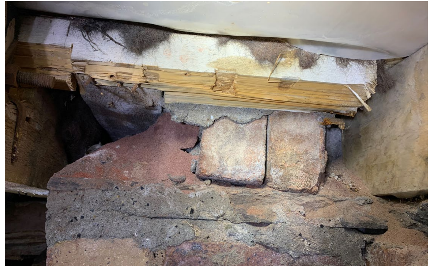
Powdered brick and stone at base of external walls in solum, 2021
