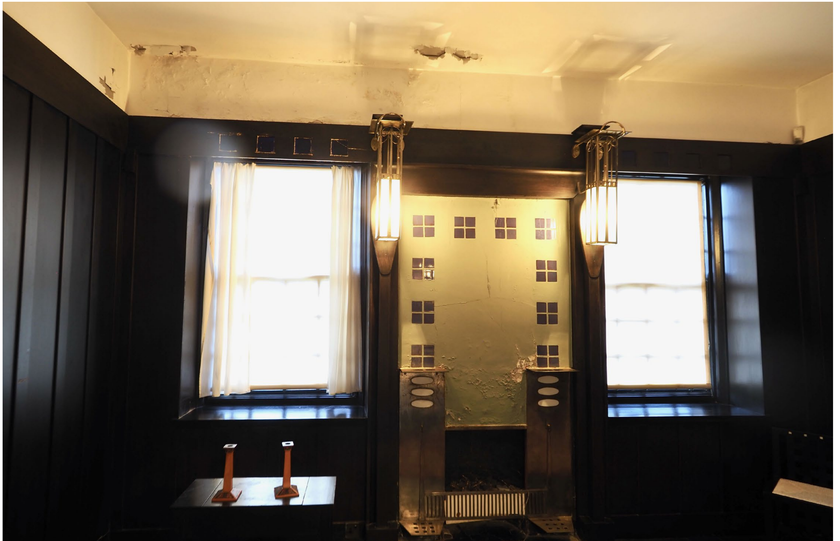
92 Dining Room showing water ingress through external wall and possible wet bridges in fabric at first floor level as well as chimney flue
