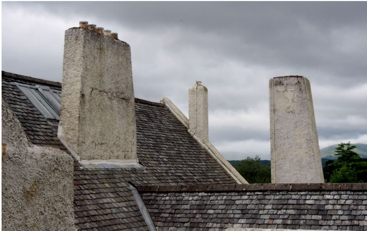
Roughcast on chimneys is cracked generally
