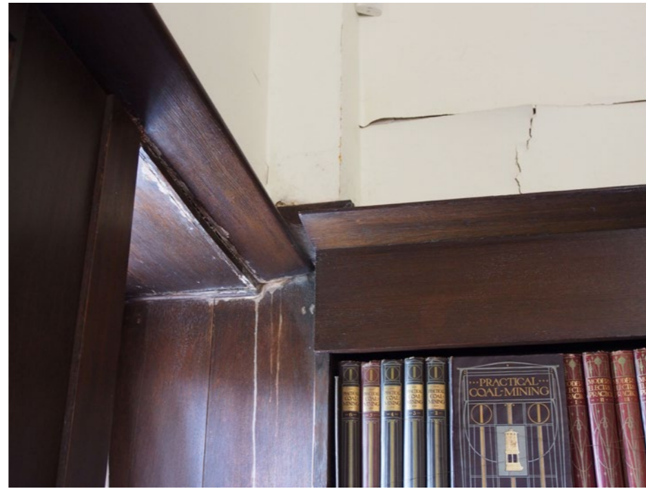
Water ingress and Damage in Library
