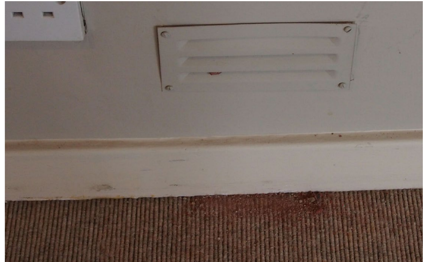
First Floor wall ventilator. Powdered brick / stone dust can be seen blown out on to carpet, 2021
