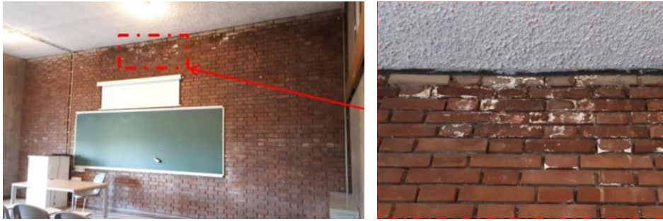
Figure 14: Salt deposits in the form of efflorescence on interior surfaces of exterior brick walls and subflorescence causing material loss on brick surfaces that progresses in time in the forms of flakes, scales and outbursts which are mostly observed at upper parts of the building where the reinforced concrete roof parapet and brick wall are in contact with each other. That signals the roof drainage faults are causing water penetration into the brick units.
