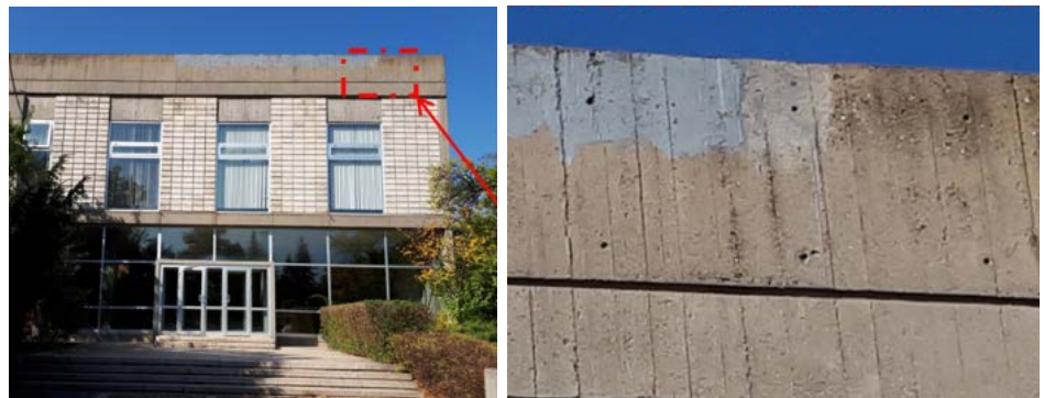
Figure 12: Dark-grey and yellowish staining on exposed concrete surfaces of the roof parapets that are continuously-washed with rainwater and partially coated with grey-colored paint to cover graffiti.
