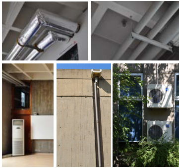
Figure 107: Additional heating pipes and AC units in the F block.
