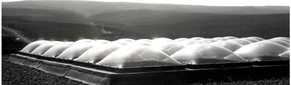
Figure 9: Transparent plastic glazing, used for skylight.
