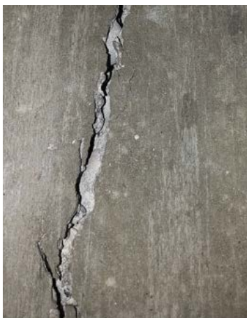
Figure 32: Close-up picture of vertical crack at the base of waffle beam.
