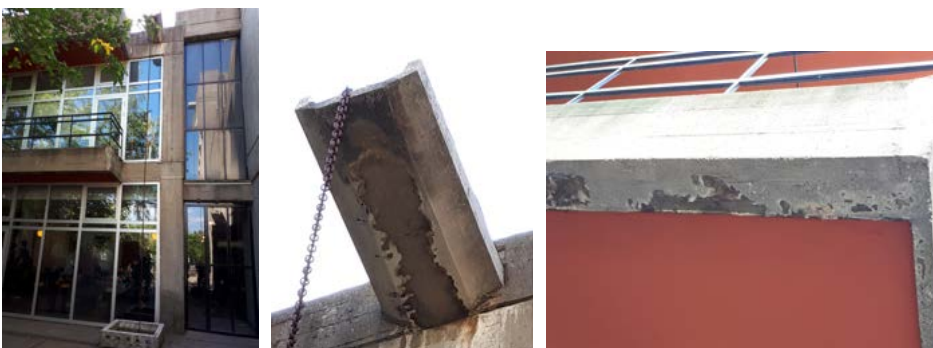
Figure 5: Material loss in concrete at the bottom surface of a waterspout and balcony edges in the form back weathering due to exfoliation (on the right top) and flakes (on the right bottom). Salt deposits are visible on those concrete surfaces.
