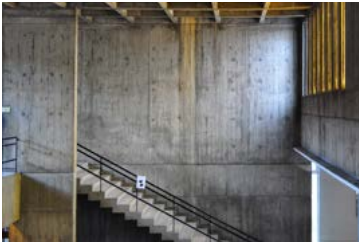
Figure 81: Molding traces and the lap joint lines.
