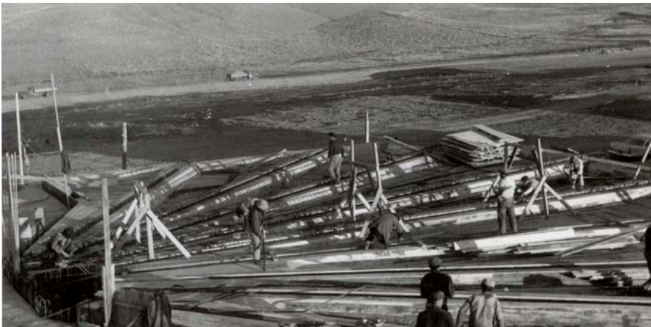
Figure 21: Construction process of METU Faculty of Architecture Amphitheater, SALT Research, Altuğ-Behrüz Çinici Archive. “There should be no more than 50-80 cm between the funnels used in the curtain castings.” 11
