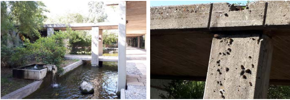
Figure 2: Material loss in concrete at the parapet of the arcade in the form of outburst together with depositions as biological growth on exposed concrete surfaces in the forms of moss and lichens (yellow-colored surfaces).
