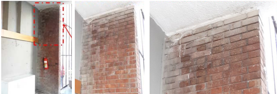
Figure 15: Salt deposits in the form of efflorescence on interior surfaces of exterior brick walls which are mostly observed at the edges where reinforced concrete exterior wall and brick wall are in contact with each other. That signals water penetration into the brick units through the edges which causes transfer of sulphate salts in cement jointing mortars to the brick body.
