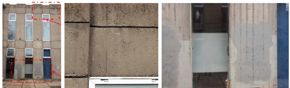
Figure 13: Dark-grey staining and microbiological growth on exposed concrete parapet surfaces in the forms of dirt patina and lichens (yellow-colored surfaces) (on the right top). And grey paint in several layers applied to cover/hide the graffiti (on the right bottom).
