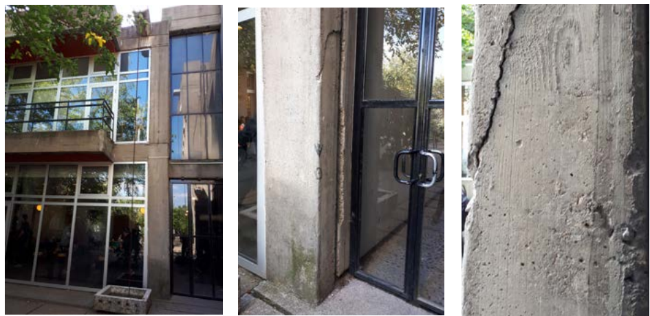
Figure 16: Diagonal crack observed in the exposed concrete shear wall at the ground floor of the building which may be due to differential settlement movement over time while the expansion joint seemed to provide complete separation between two shear walls since no cracks are observed at the neighboring shear wall.
