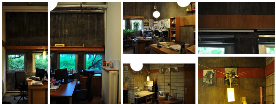
Figure 108: Remains of the exposed concrete surfaces and wooden bands in the F block
