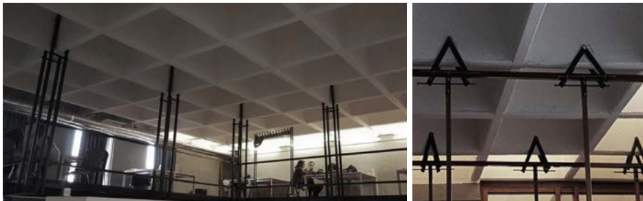
Figure 9: Different types of mezzanine hanger bars attached to the waffle slab of one of the 3rd year design studio, designed by a former instructor, Arda Düzgüneş.
