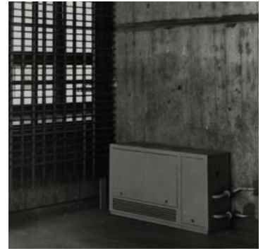
Figure 11: Original Fan coil units.
