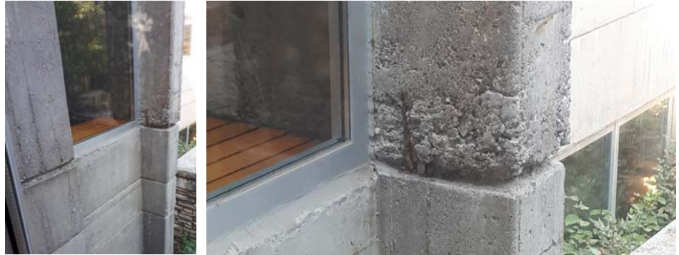
Figure 7: Material loss at the edge of structural reinforced concrete column in the forms of aggregate loss, surface roughening and edge rounding that results in exposure of reinforcement bars to atmospheric conditions and their corrosion.
