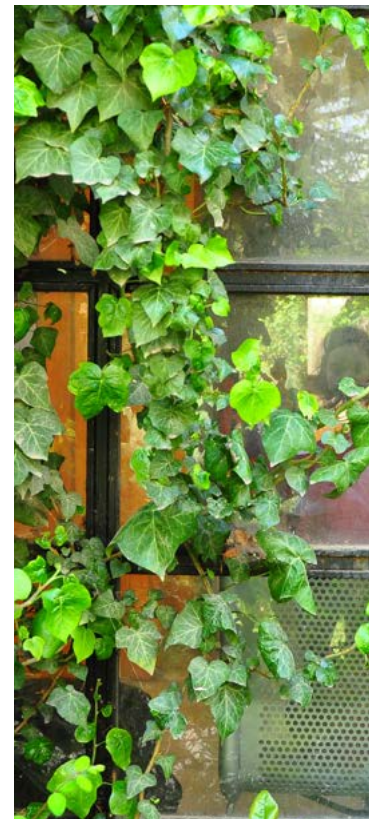
Figure 24: Iviens on the curtain wall of the industrial design studios
