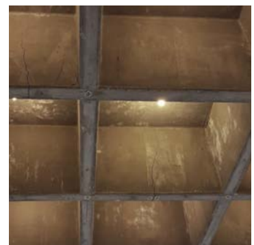
Figure 8: Positive bending moment related tension cracks in the 1st floor waffle slab of the selected part of the building.
