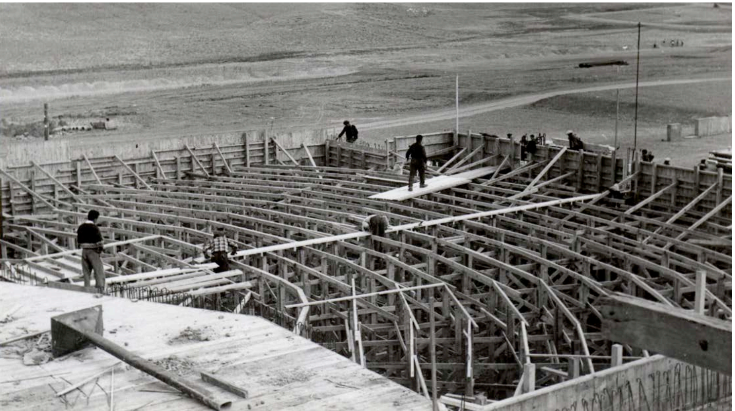
Figure 20: Construction process of METU Faculty of Architecture Amphitheater, SALT Research, Altuğ-Behruz Çinicici Archive
