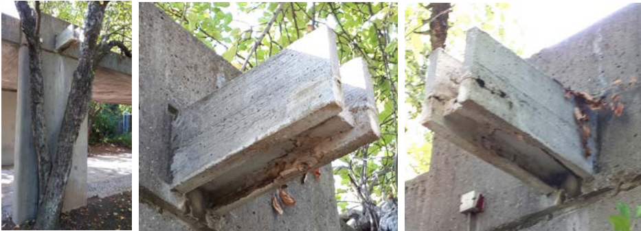
Figure 3: Material loss in concrete at waterspout in the forms of outburst, which results in exposure of the reinforcement bars to atmospheric conditions and their corrosion. Material loss associates with detachments in the form of flakes together with longitudinal cracks and deposits as biological growth in those cracks and salt deposits on deteriorated concrete surfaces.
