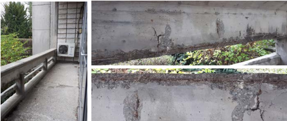
Figure 4: Material loss in concrete at exposed balustrades in the forms of outburst and aggregate loss which results in exposure of reinforcement bars to atmospheric conditions and their corrosion. Detachment on exposed concrete surfaces in the form of crumbling and flakes showing that such detaching surfaces are areas that are at risk of, loss and require urgent intervention.
