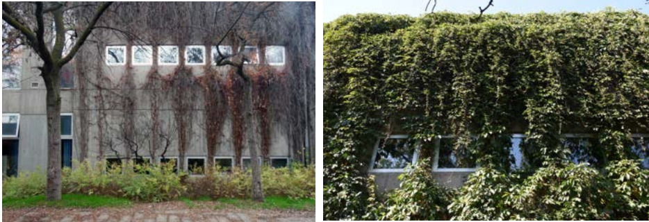
Figure 110: Current condition of the east façade of the F block, ivy growth respectively in fall and spring.
