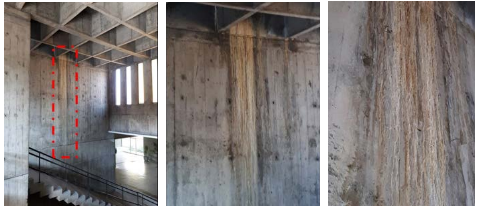
Figure 11: White and yellow discoloration on exposed concrete surface signaling the local dampness problem at the upper part of the building due to the roof drainage fault resulting in water seepage through the roof level. The presence of salt deposits with yellowish color staining indicates that the reinforced concrete roof slab suffers from continuous dampness problem and corrosion of reinforcement.
