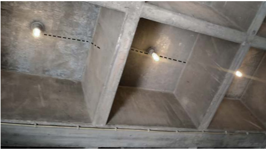
Figure 30: Negative bending moment region and tension cracks at the slab level.
