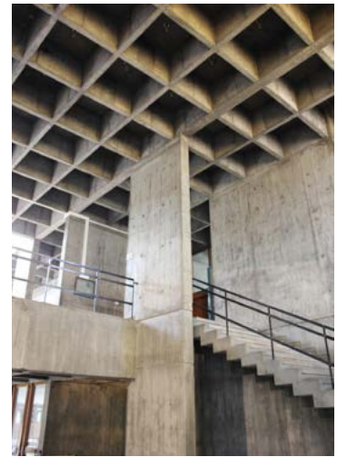
Figure 6: Waffle slab to column connection at the selected part of the building.
