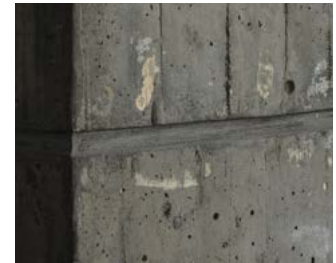
Figure 120: Joint gap lines
