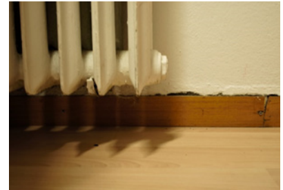
Figure 129: Wooden skirting inserted in recessed surface
