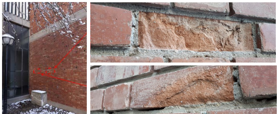
Figure 8: Material loss rarely observed at exposed brick masonry units in the form of outbursts together with detachments in the forms of flakes and scales.
