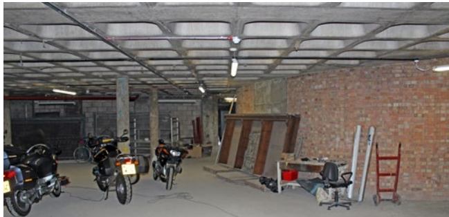
A view of the large scale open areas in the Gibberd podium, accessed off the car park, that are used for storage
