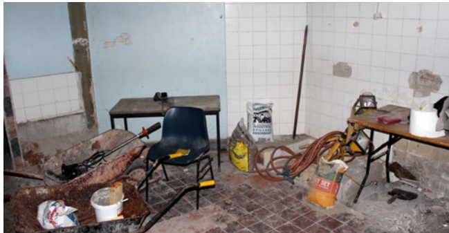
Part of the large scale spaces on the western side of the Gibberd podium
