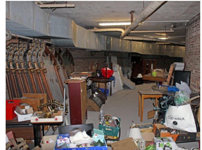
The outer room of the central drum showing the service ducts to the ceiling and the storage
