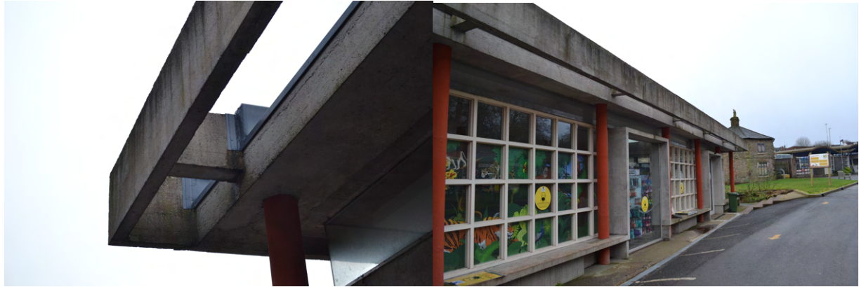
Fig 34 & 35. Image of the false fascias on the former Station Cafe, taken on 4th February 2021
