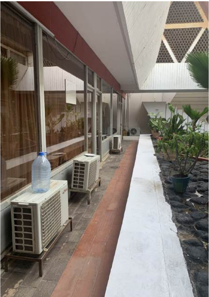
Fig.73: ( top) air conditioning units are endemic to the facades of the offices in the innovation centre. This is mostly due to passive climate strategies being defunct and overcrowding (photo: Dana Salama, 2021).
