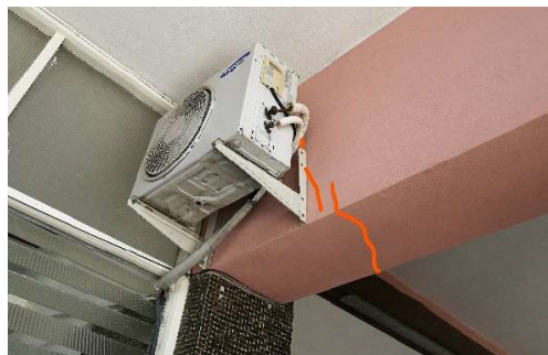
Figure 4.57 Deformation and cracks of the columns of the platform's area.
