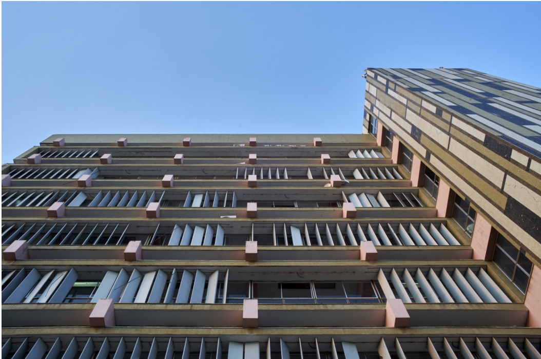
Figure 5.8 Main façade of the administration block showing missing Brise-soleil (EM, 2019).
