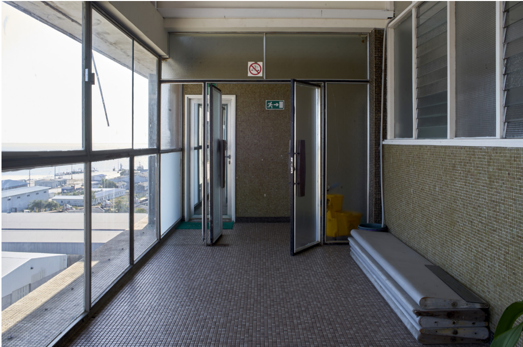
Figure 5.10 Brise-soleil from the main façade of the administration block torn off by Hurricane Idai (EM, 2019).
