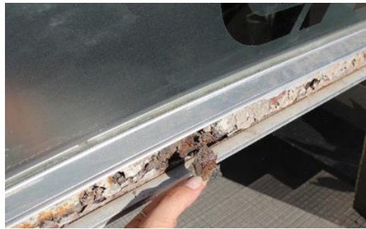
Figure 4.52 Detachment of the sun protective system on the front façade of administration block.
