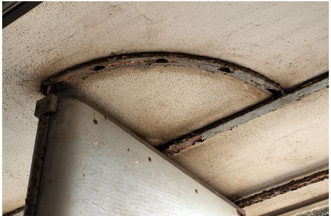
Figure 5.9 Brise-soleil mechanism showing corrosion (EM, 2009).
