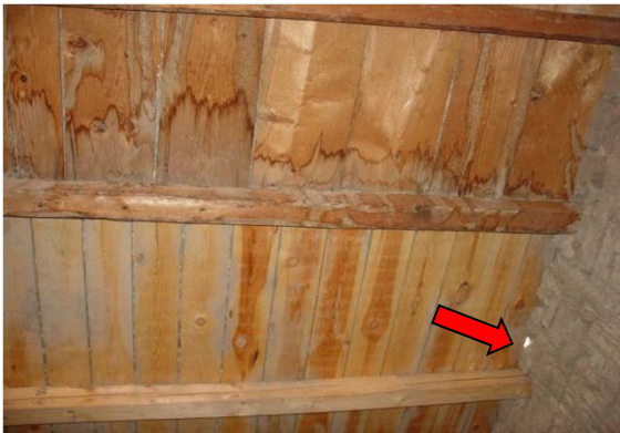
Interior view of water stains on the wooden ceiling adjacent to the hole in the roof (arrow).
