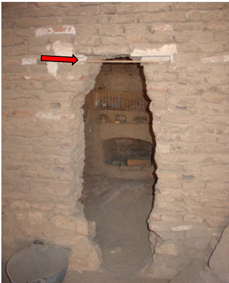
View of missing lintel (arrow) in doorway between the northeast room and the west room.
