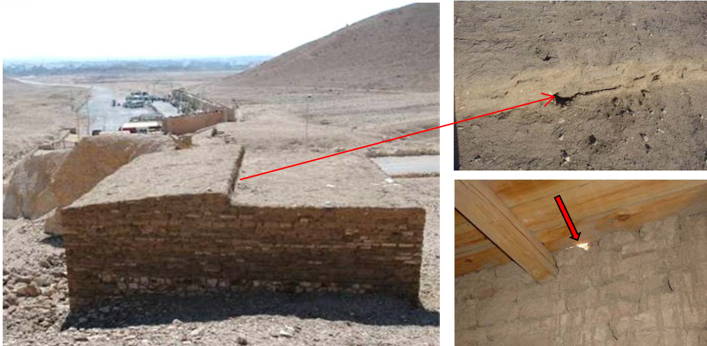
Left: North elevation with site entrance and parking area in background. Upper right: Detail of the hole in the building's roof at the juncture between the two levels. Lower right: Interior view of the hole in roof (arrow), with mud drip lines below providing evidence of water infiltration.
