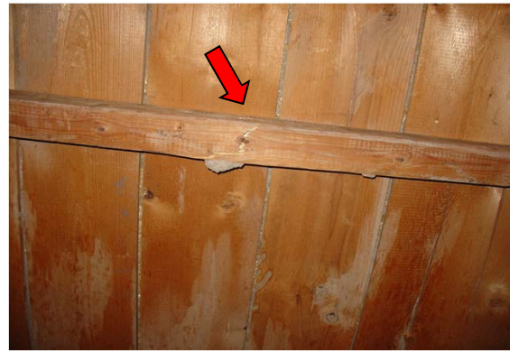
Crack in the middle of the beam supporting the roof in the southeast room. The roof sags in this area.
