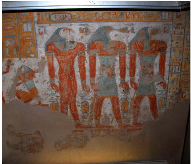
Loss of painted plaster at the wall base of tomb QV 52 (Tyti) presumably due to historic flooding. The tomb, open to general visitation, is in a vulnerable position near the main drainage channel.
