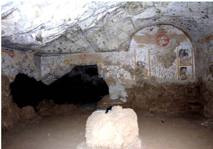
Rock collapse, deterioration, and loss of painted plaster in the lower walls of tomb QV 60 (Nebettauy) due to repeated flooding, including in 1994.
