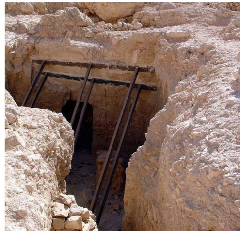
View of roof collapse of tomb QV 34, which is in an area where most tombs contain shale susceptible to water damage.
