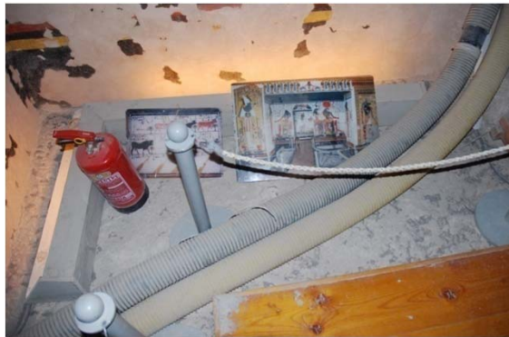
Fire extinguisher and air extraction pipes in upper chamber. Contact of pipes with wall causes abrasion.
