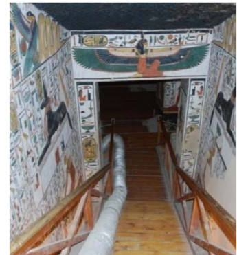
Large extraction pipe from lower chamber.
