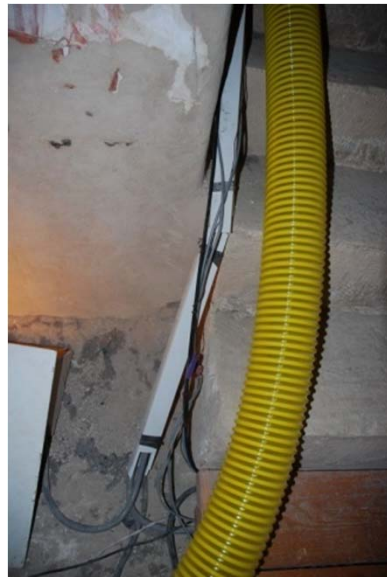
Electrical wiring from the junction box into Chamber C was encased in conduits.
