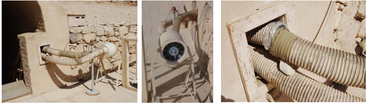
Air extraction pump outside entry to tomb. The pipe exits at the front of the tomb and is a significant visual intrusion. Extraction pipe was broken in several places, occasionally repaired with tape.
