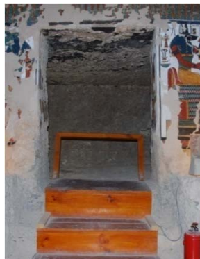
Walkway barriers are low and too close to wall paintings at doorways. Barrier to Chamber Q (above) is not stable.
