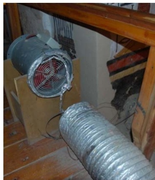
Broken extraction pipe at top of stairs.
