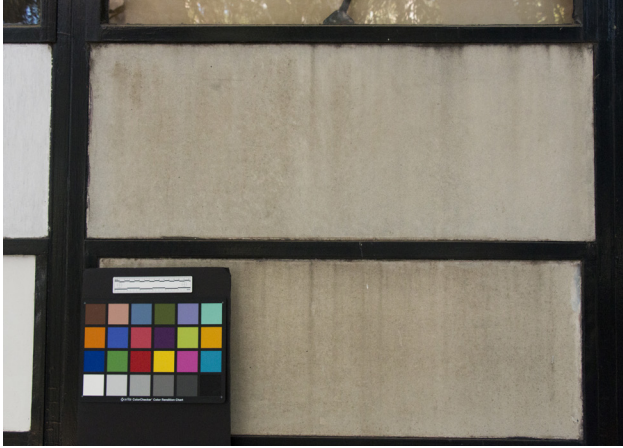
FIGURE 3.3 Photo of Eames residence exterior, east elevation, showing heavy soiling on panels HE-8-5 and HE-8-6. Photo: Laura Matarese and Chandler McCoy, 2015. ©J. Paul Getty Trust.
