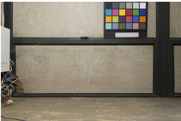
FIGURE 3.7 The letter B written in chalk in the center of the asbestos-cement facing of a lower panel in the Eames studio interior. Note broken lower left corner, possibly caused during the installation of telecommunication and internet wires. Photo: Laura Matarese and Chandler McCoy, 2015. ©J. Paul Getty Trust.
