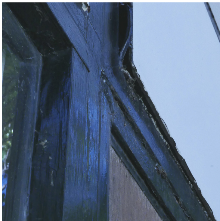
FIGURE 3.12 Panel on the residence exterior, north elevation, damaged after heavy rainfall in 2017. The outer asbestos-cement facing has been pushed out and detached from the Celotex fiberboard core, adhesive, and outer sealant. Photo: Laura Matarese and Chandler McCoy, 2017. ©J. Paul Getty Trust.
