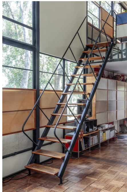
FIGURE 2.2 View of the interior faces of the Cemesto and replacement panels (painted and unpainted) shown in figure 2.1. Note the open-tread staircase that partially conceals them and the Plyon window panels in custom-designed wooden frames that provide light control. Photo: Joshua White, 2016. ©Eames Office.
