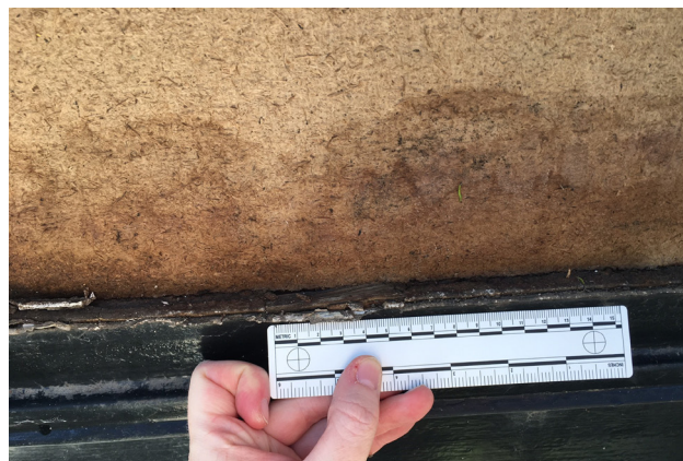
FIGURE 3.14 Panel SE-11 in 2017, showing damage after heavy rainfall. The Celotex fiberboard core, exposed when the exterior asbestos-cement facing fell off, was saturated with water. Wood shims were found to have been installed around the panel to hold it in place, as shown here under the exposed core. Photo: Laura Matarese and Chandler McCoy, 2017. ©J. Paul Getty Trust.
