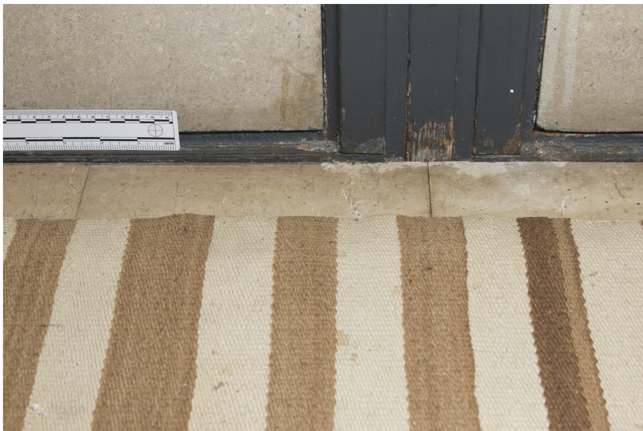
FIGURE 3.11 Example of rust in the lower corners of a steel frame surrounding Cemesto panels. Photo: Laura Matarese and Chandler McCoy, 2015. ©J. Paul Getty Trust.
