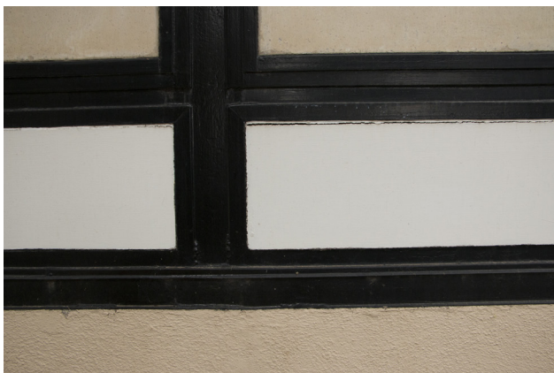
FIGURE 3.13 Panel SE-11, studio exterior, east elevation, in 2015, prior to detaching and falling off in 2017. Note the signs of cracking and breaking away at the top of the panel. Photo: Laura Matarese and Chandler McCoy, 2015. ©J. Paul Getty Trust.
