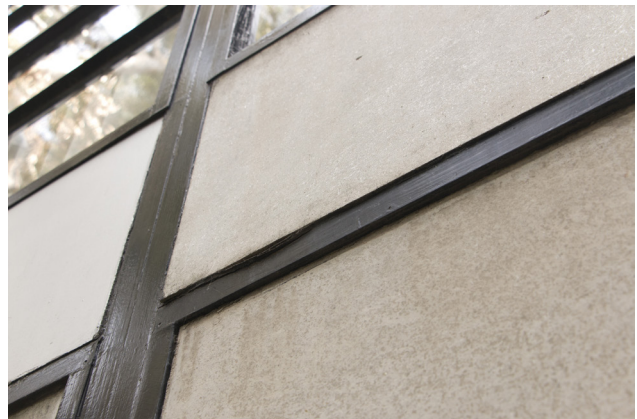
FIGURE 3.10 Panel on the residence exterior, north elevation, showing the outer asbestos-cement facing detaching from the fiberboard core and sealant on the lower corners. Photo: Laura Matarese and Chandler McCoy, 2015. ©J. Paul Getty Trust.
