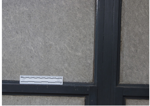
FIGURE 3.4 Photo of Eames House studio interior, east elevation, showing no soiling and the natural mottled gray color of the asbestos-cement board. Photo: Laura Matarese and Chandler McCoy, 2015. ©J. Paul Getty Trust.
