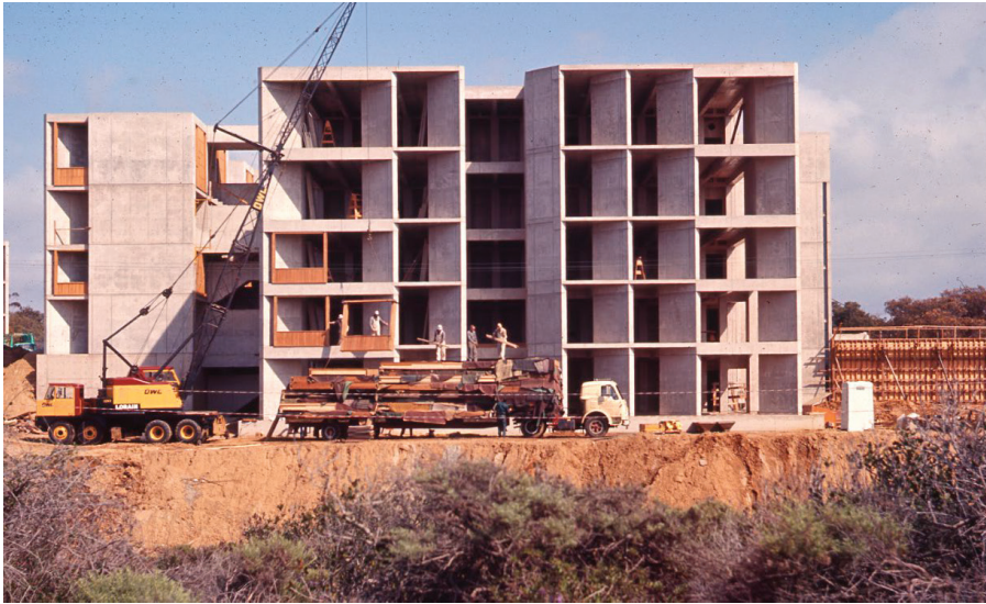
FIGURE CS-B.3 View of the southern west office wing, with prefabricated window walls being installed, circa 1965. Image: Louis I. Kahn Collection, University of Pennsylvania and Pennsylvania Historical and Museum Commission, scan 030.V.D.19.2_Mar65.
