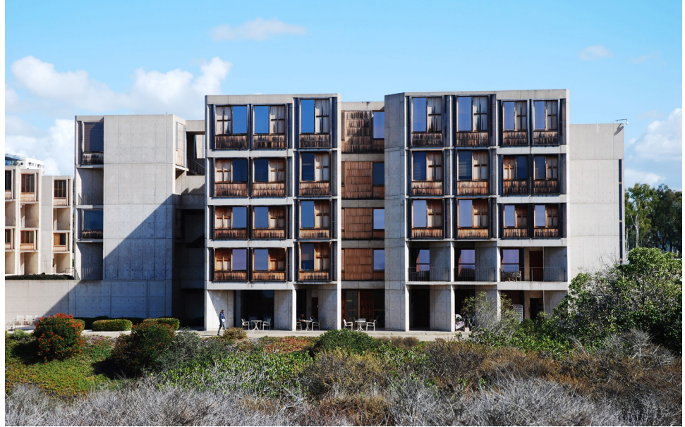
FIGURE 15. West-facing elevations of the Salk Institute, showing a black fungal biofilm at the base of the teak window wall assemblies prior to conservation efforts, 2014.
