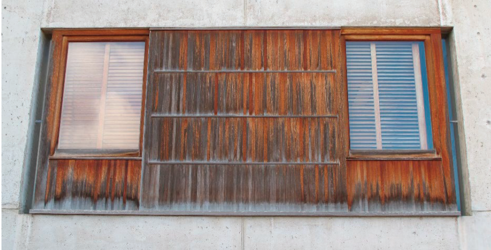
FIGURE CS-B.6 View Mock-Up 1.A (Minor intervention with in situ cleaning and repair, with investigation and treatment of interior framing), prior to treatment, September 18, 2014. Photo: J. Paul Getty Trust
