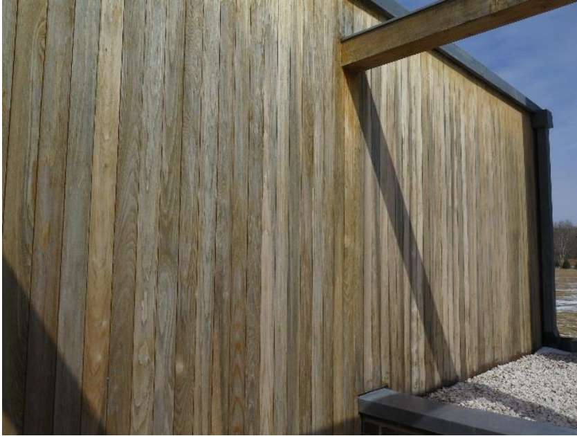
FIGURE CS-C.5 Elevation showing the cypress siding, with surface treatments removed, in the process of weathering, February 2015. Photo: J. Paul Getty Trust
