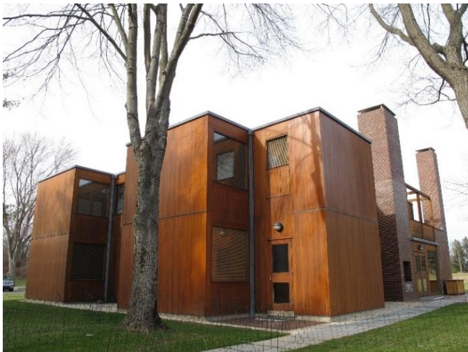
FIGURE CS-C.2 Photograph showing past surface treatment of the exterior wood siding, with a dark orange color, April 2014. Photo: J. Paul Getty Trust
