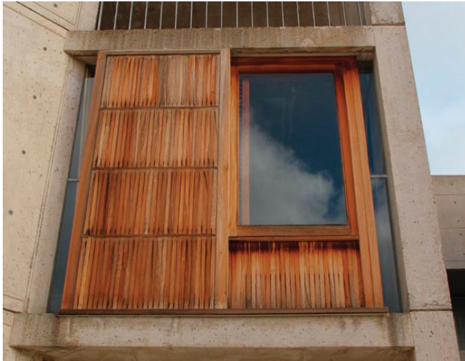
FIGURE CS-B.11 View of Mock-Up 3 (replacement of severely deteriorated window wall with in-kind materials) prior to treatment, September 18, 2014. Photo: J. Paul Getty Trust
