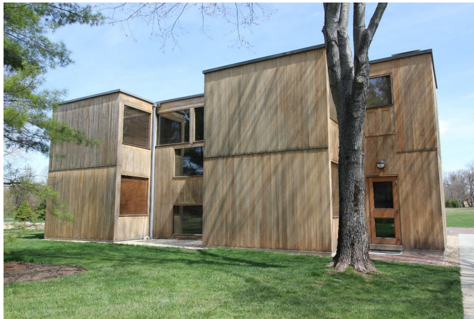
FIGURE CS-C.12 View of cypress siding during natural weathering process May 2015. Photo: Andrew Fearon
