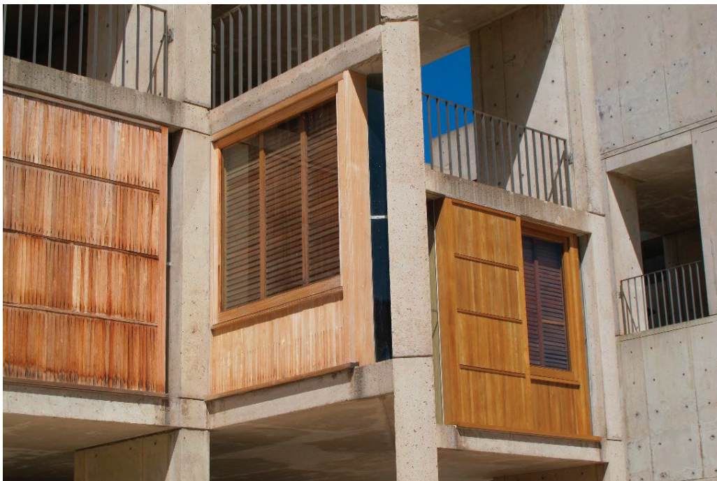
FIGURE CS-B.14 View of North Study Towers, illustrating the range of conditions extant near the completion of the trial mock-up construction activities on March 30, 2015. From left to right: Existing weathered and uncleaned south-facing teak (no work undertaken at this window wall), cleaned and brightened west-facing teak at the center (Mock-Up 1.C), and a reconstructed window wall assembly with new FEQ and reclaimed teak, facing south (Mock-Up 3). Note that the south and west-facing windows typically have a more bleached appearance than the north-facing windows. Photo: J. Paul Getty Trust
