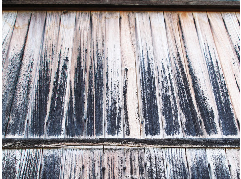
FIGURE 17. Detail view of window wall assembly, 2014. The outermost face of the intermediate horizontal drip (bottom of photo), with its ¼-inch projection, has weathered away in some areas, exposing the tops of the vertical T&G boards underneath.
