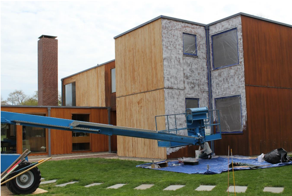
FIGURE CS-C.10 View of cypress siding during finish removal with benzyl alcohol, May 2014. Photo: Andrew Fearon
