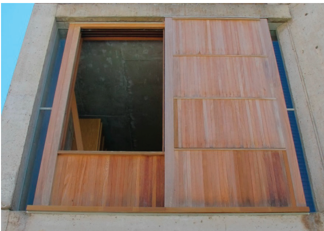
FIGURE CS-B.10 View of Mock-Up 2, near completion of treatment, March 30, 2015. Similar cleaning and surface treatments to Mock-Up 1.A were also carried out at Mock-Up 2. In addition, the use of an oxalic acid based brightener was used, which removed the moisture stains remaining after cleaning. Performance-based improvements included trimming the ends of the T&G boards in situ (by 1/8" or 3/16") to reduce moisture uptake through the end grains and installation of head and modified base flashings. Photo: J. Paul Getty Trust
