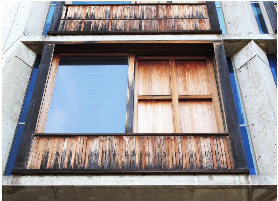
FIGURE 16. Teak window wall assemblies at the Salk, showing fungal biofilm on the wood, 2014.
