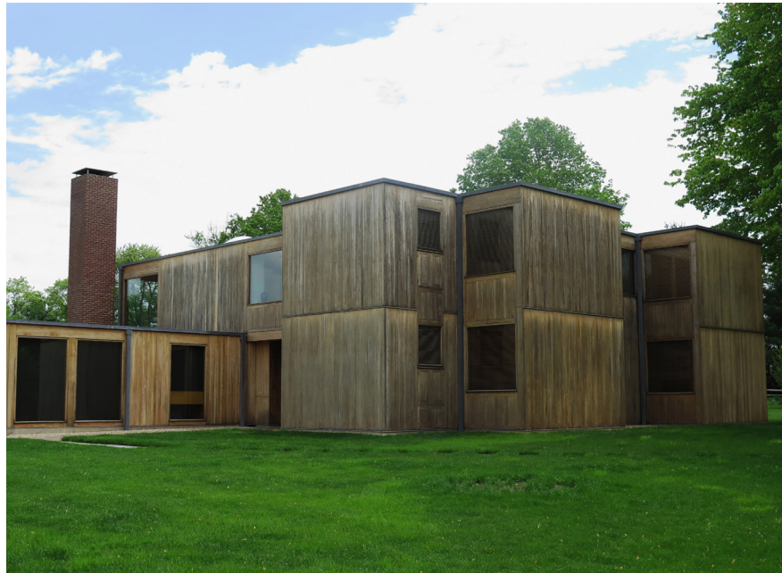
FIGURE 4. View of the Korman House from the west during the conservation project, 2015.
