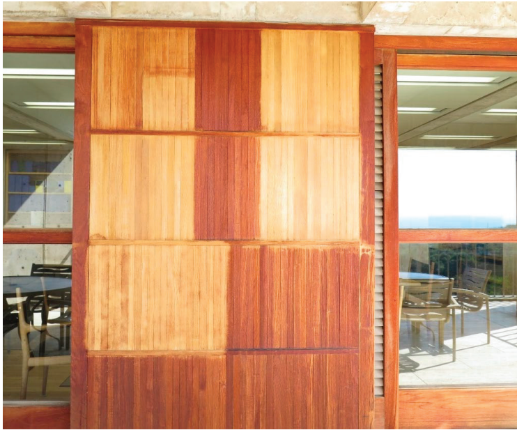
FIGURE CS-B.8 View of Mock-Up 1.B (stripping tests only), at completion of treatment, February 17, 2015. Investigations included trialing various non-toxic or low-toxicity chemical and mechanical strippers to remove past surface coatings. Clockwise from top left: mechanical sanding (150 grit) and partial 3M Safest Stripper Paint and Varnish Remover; Soy Gel Professional Paint Stripper; Citristrip Safer Paint and Varnish Gel; Sponge-Jet Sponge Media for Sensitive Substrates (White Media Sponge, profile of <6microns) Jet; and 3M Safest Stripper Paint and Varnish Remover only. Photo: J. Paul Getty Trust
