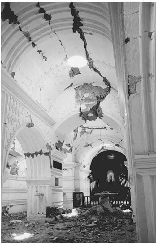
The heavily damaged 18th-century vaulted masonry church of Nuestra Señora del Pilar, one of the few existing examples of Baroque architecture in El Salvador. Photo: Mary Hardy.
