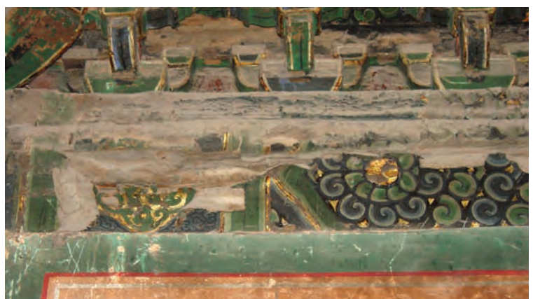
大额枋上剥离下垂的彩画局部。 Detached and falling area of painting on the architrave.
