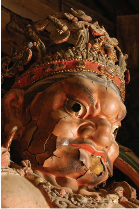
“哼”头部细节，可见严重开裂及油饰地仗层的缺失。 Detail of head of Temple Guardian Heng showing severe cracking and loss of the painted plaster layer.
