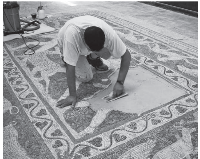
FIGURE 4 Application of lime mortar in a neutral color used to replace the black cement. Photo by Robert (Chip) Vincent.
