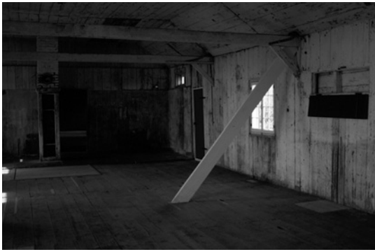
The interior of the east end of the Lazaretto, showing one of the diagonal braces as well as one of the windows modified for a late use of the building.
