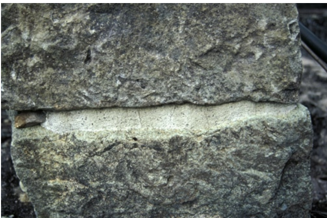
Figure 103 Lime-based mortar mix with added pumice, made in February 2005, shown after ten months of unsheltered exposure at the top of the Stairway. December 2005.
