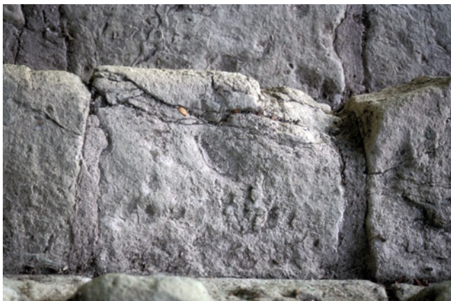
Figure 140 An in situ block (step 10, block 55) tread surface seen from above; the parallel cracks are behind the carved block face.
