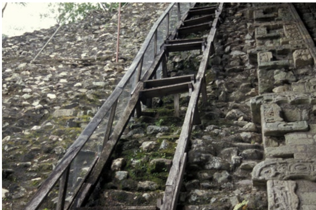
Figure 155 Area of increased biological growth near the Stairway, where rainwater flows toward it.
