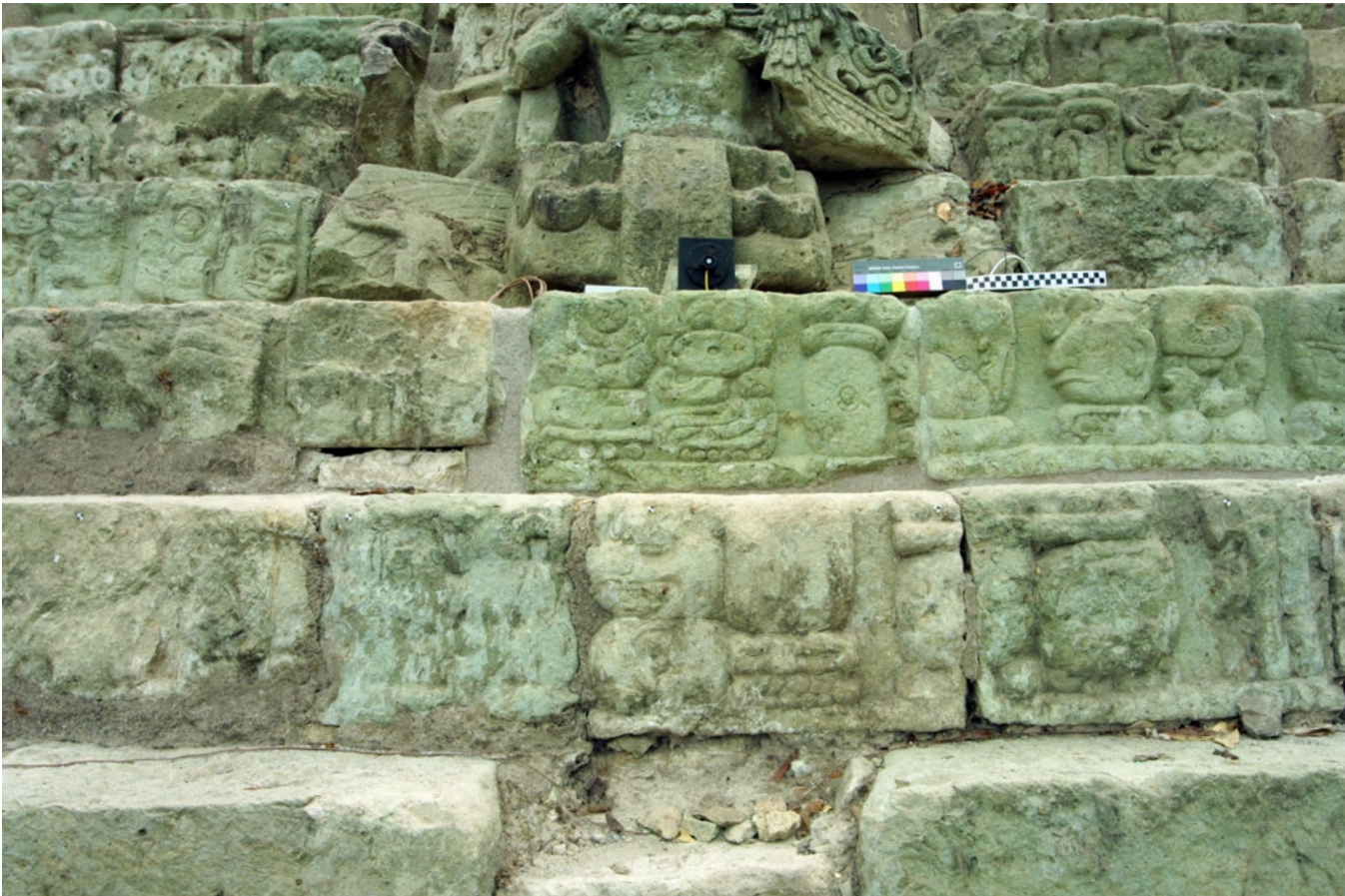
Figure 145 A view of step 42, in the foreground, shows missing repointing mortar (right) and previous repointing, where mortar covers edges of the blocks (left).
