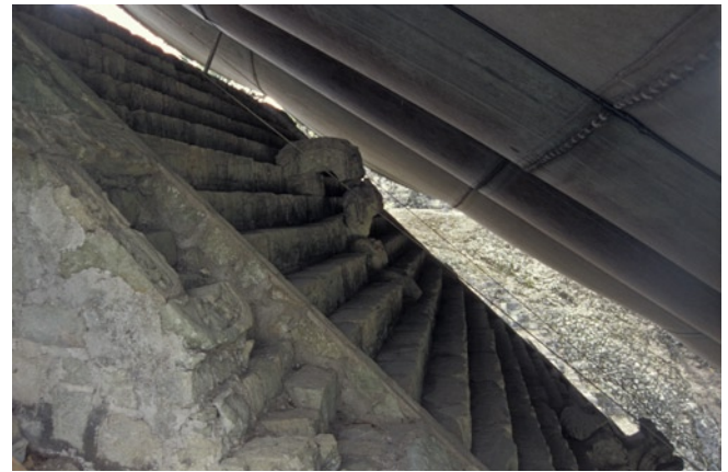
Figure 130 Shelter in 2000; note the proximity of the tarpaulin to the top of the Stairway.
