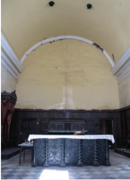
FIGURE 4.59 Sector F: The upper west wall behind the altar exhibits out-of-plane displacement and cracking. Image: Sara Lardinois.
