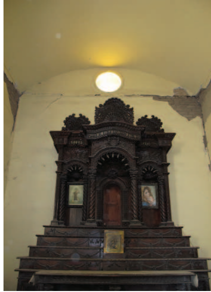
FIGURE 4.60 Sector F: View of vertical cracking in either corner at west wall of the north side chapel, behind altarpiece B. Image: Sara Lardinois.
