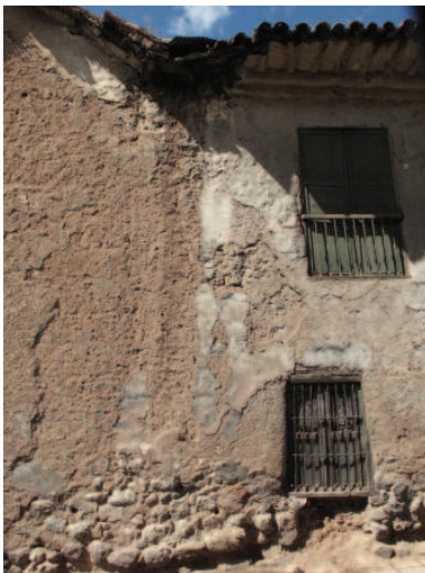
FIGURE 6.40 Erosion and loss of base course stones outside room C-109, north façade. Image: Claudia Cancino.
