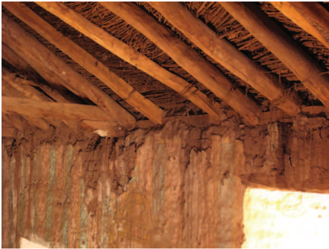
FIGURE 5.31 View of rafters and wall plate at the lateral wall of nave. Image: Claudia Cancino.
