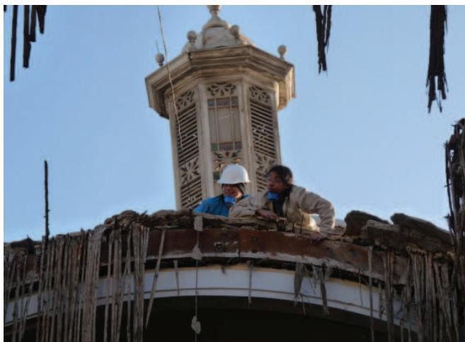
FIGURE 7.3 Prospection process: project team documenting the roof connections at the Cathedral of Ica, taking advantage of those areas made visible by the previous collapse of portions of the roof. Image: Mirna Soto, for the GCI.
