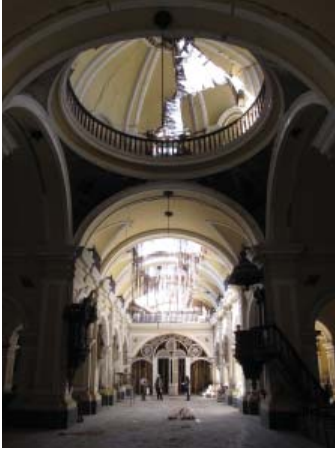
FIGURE 4.3 View of damages to the dome and vault resulting from the 2007 earthquake.
