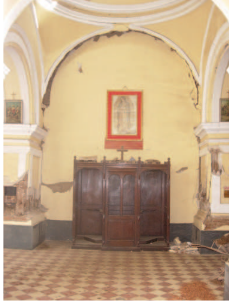
FIGURE 4.46 (LEFT) Sector B: Cracking and partial collapse at arches at the top of the wall, confessional space, 2007. Image: Philippe Garnier.
