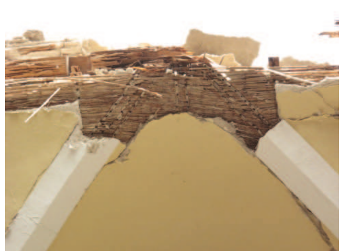
FIGURE 4.51 (TOP) Sector C: Damage to wood arches forming the nave barrel vault, with corrosion at the nails connecting the arch segments. Image: Claudia Cancino.
