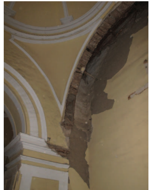
FIGURE 4.48 Sector B: Detail of cracking and partial collapse at arches along the south lateral wall. Image: Sara Lardinois.
