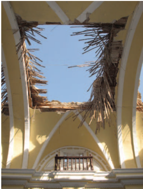
FIGURE 4.50 Sector C: View of a collapsed bay of the nave barrel vault. Image: Sara Lardinois.
