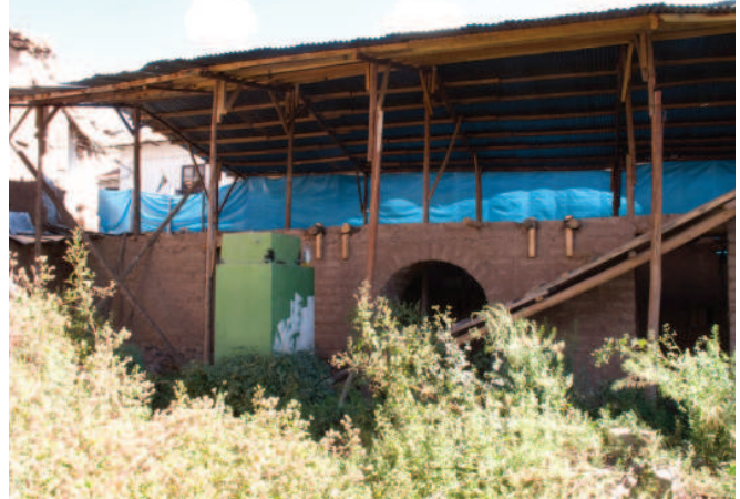
FIGURE 6.6 Collapsing rear wing of house along Calle Nueva Alta (not part of construction assessment), with shoring and temporary roof in place. Image: Amila Ferron.
