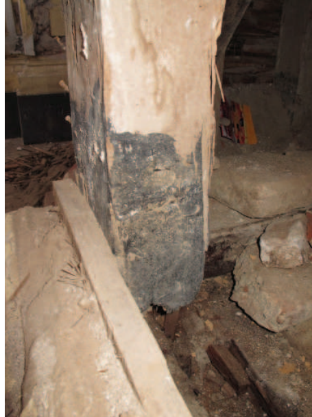
FIGURE 4.53 (NEAR RIGHT) Sector C: View of pillar base, showing deterioration of the wood post and sill. Image: Sara Lardinois.
