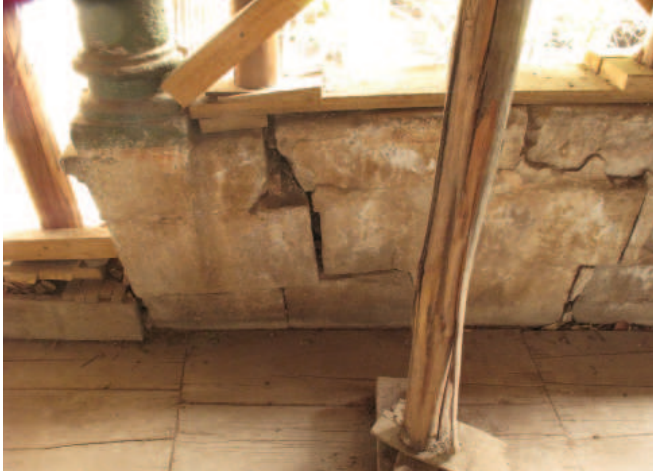
FIGURE 6.46 West end of stone masonry parapet wall at south arcade, as viewed from room B-206. Image: Sara Lardinois.
