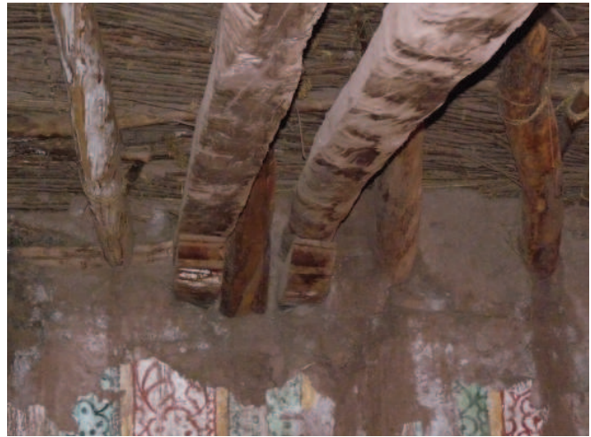
FIGURE 5.32 View of the pair of tie beams over the nave. Image: Mirna Soto, for the GCI.
