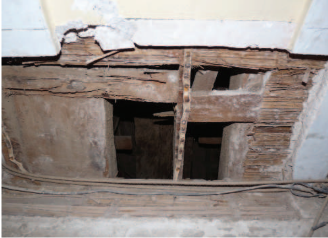
FIGURE 4.32 (ABOVE LEFT) View of plaster and caña chancada (flattened cane reeds) at the interior side of the vault. Image: Mirna Soto, for the GCI.
