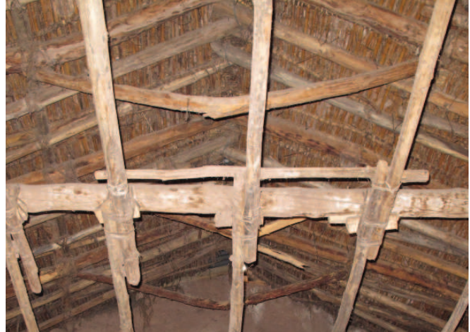
FIGURE 6.48 View of broken collar ties. Image: Sara Lardinois.
