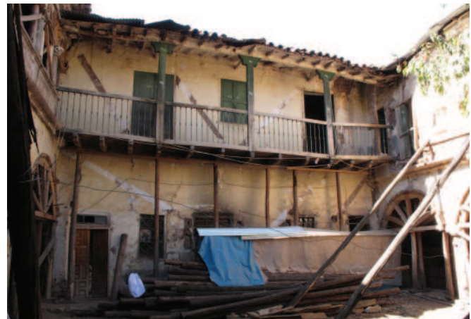
FIGURE 6.14 View of cantilevered wood balcony at east side of patio. Image: Sara Lardinois.
