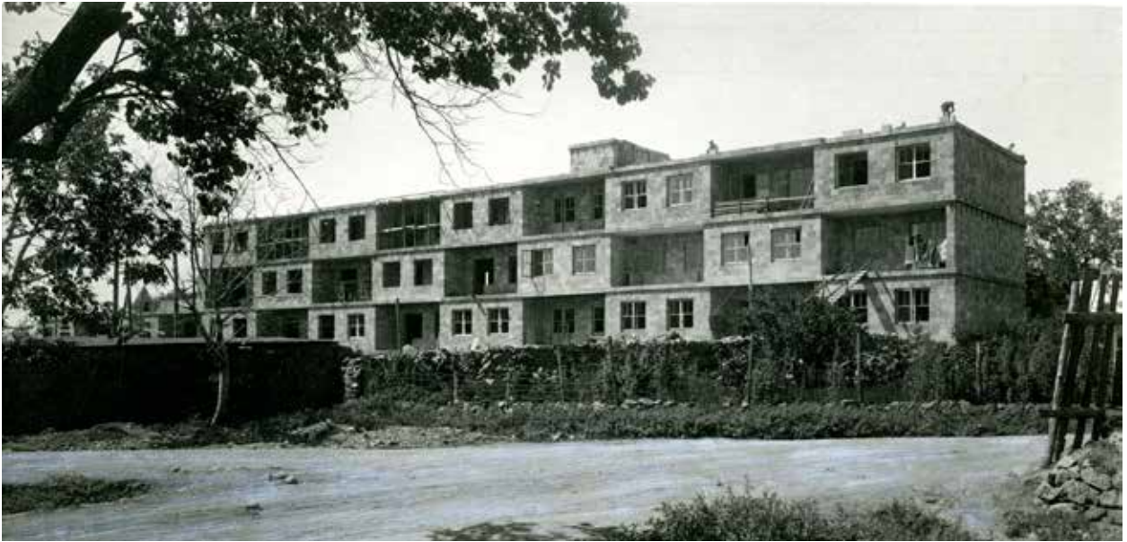
Picture 21. Residential building for workers of the hydroelectric power station in Yerevan, the so called "Chess house", 1931
