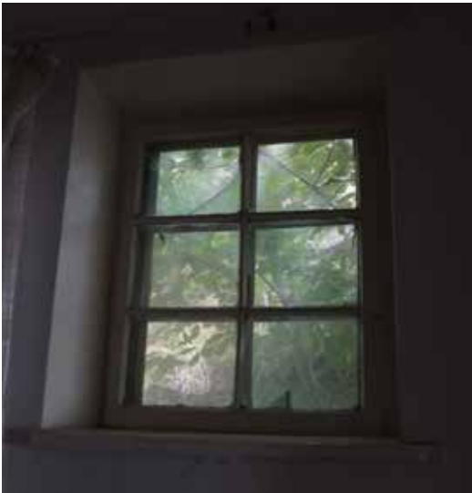
Picture 96. Window on the second floor dated 1936, 2016. Photo by Sarhat Petrosyan
