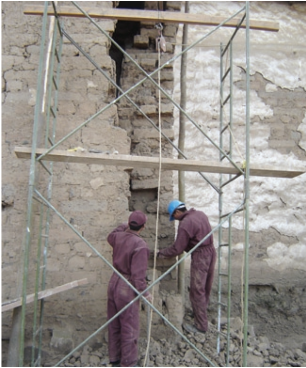
FIGURE 10 Damaged corner in the process of being demolished and rebuilt, San Pedro de Navan.
