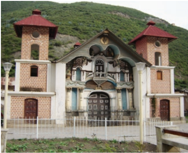
FIGURE 4 Incompatible materials used at Huacho sin Pescado Missionary Chapel.
