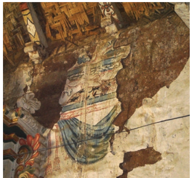
FIGURE 3 Moisture damage at the top of the walls, Rapaz Missionary Chapel.
