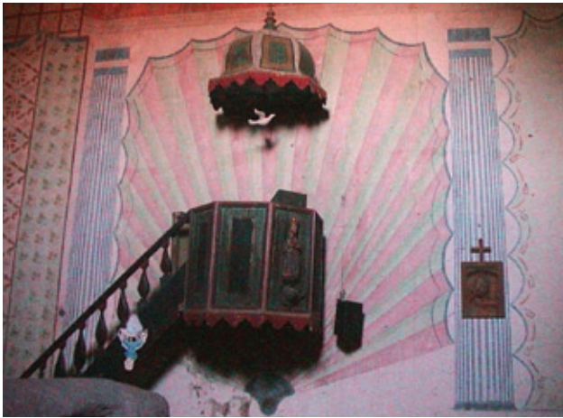
FIGURE 3 Interior of Mission San Miguel Chapel after the 2004 San Simeon earthquake. The decorative interior wall finishes were badly damaged. Photo: E. Leroy Tolles, ELT and Associates.
