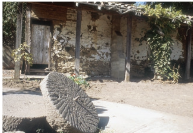
FIGURE 5 Don Jose Antonio Bolcoff Adobe, ca. 1840, Wilder Ranch State Park, near Santa Cruz, California. The Bolcoff Adobe's deteriorated condition is the result of deferred maintenance. Photo: California State Parks, © 1988.
