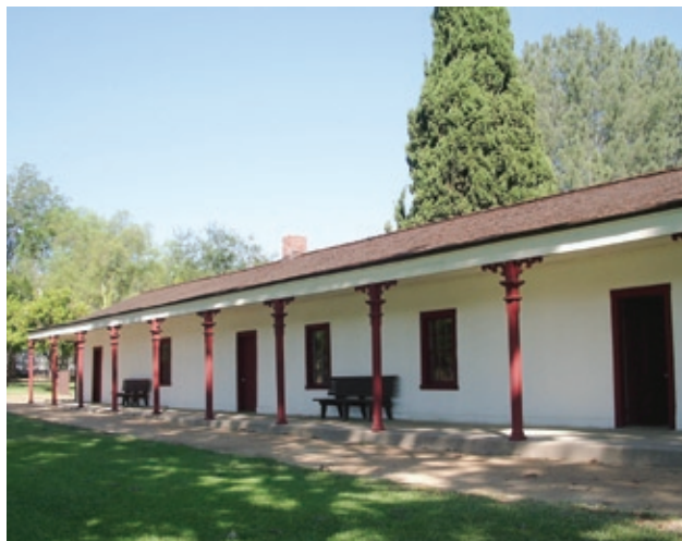
FIGURE 6 Exterior of de la Ossa Adobe, Los Encinos State Historic Park, Encino, Los Angeles. The adobe was damaged by the 1994 Northridge earthquake. Photo: Courtesy of Karen Hildebrand, California State Parks.
