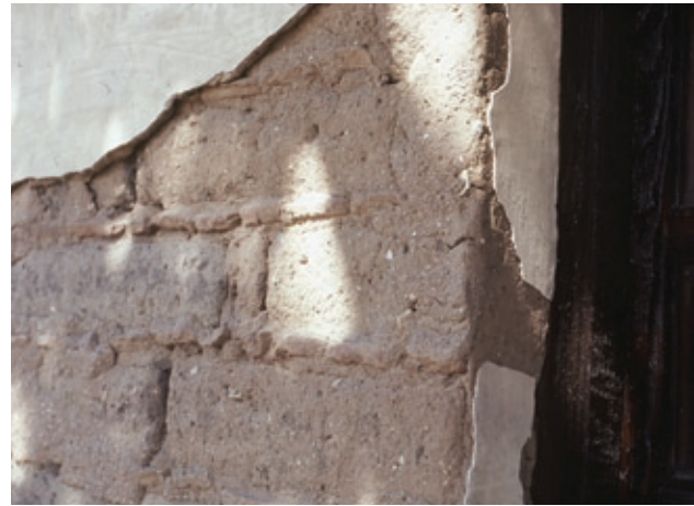
FIGURE 4 Adobe garden wall at Cooper-Molera State Historic Park, Monterey, California. Freestanding adobe structures are difficult to maintain and retrofit seismically.
