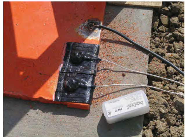
Figure 11b The cable connections to the sculpture are coated with a bituminous material to make them waterproof.
