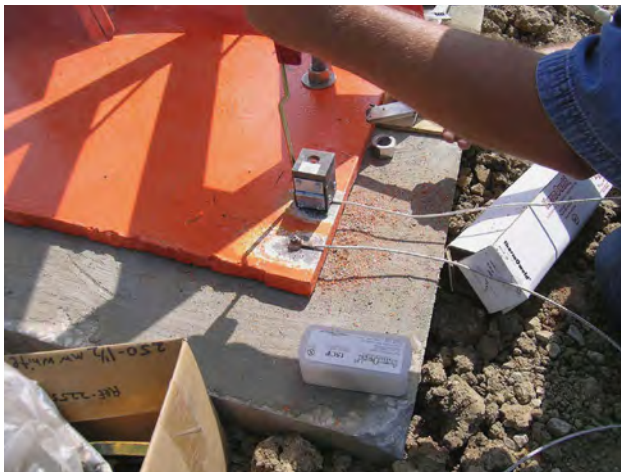
Figure 11a A thermite explosive charge is used to produce an extremely high temperature that bonds the cables instantly to the sculpture's clean metal surface.
