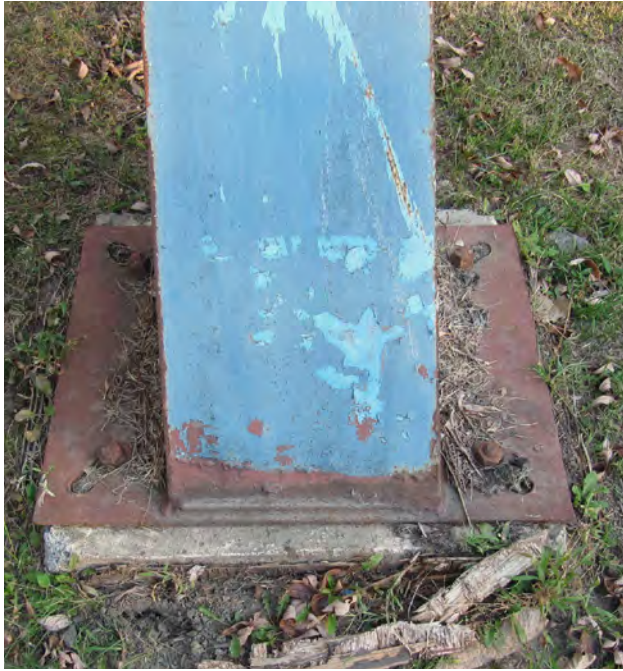
Figure 2 Example of deterioration due to improper maintenance, showing grass projections and scratches from maintenance equipment. Photo: Nathalie Richard, 2012 © CCQ.
