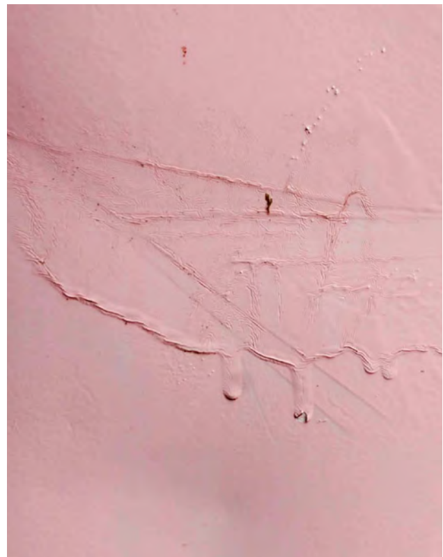
Figure 2 Detail of Flause . Drips visible in the surface structure of the paint indicate a lack of careful paint application.
