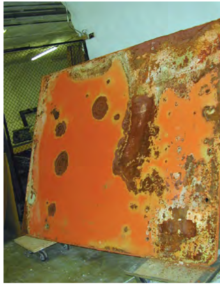
Figure 9 (Right) Bottom surface of the base plate, showing heavy rust and missing paint. (Far right) Detail of the contact area between steel beams, showing heavy rust and missing paint.
