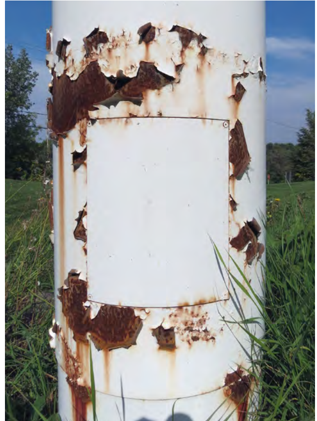
Figure 3 Example of deterioration due to improper maintenance, showing paint lifting and corrosion of steel behind the weeds. Photo: Marie-Chantale Poisson, 2012 © CCQ.
