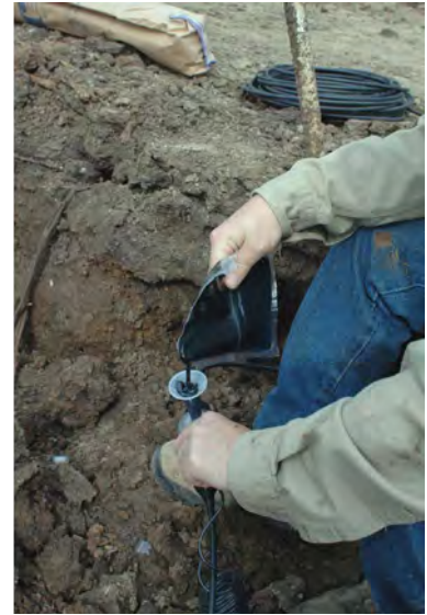
Figure 10c The cable connection housing is filled with a bituminous material to make the cable connections waterproof.
