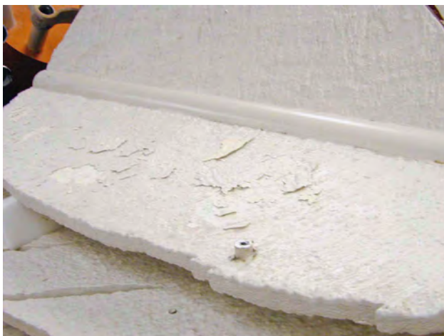
Figure 4 Flaking and lifting paint on a feather of one of the Shuttlecocks .
