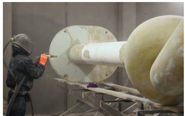
Figure 7 Sandblasting was used to remove the old paint layers. Photo: Lydia Beerkens.
